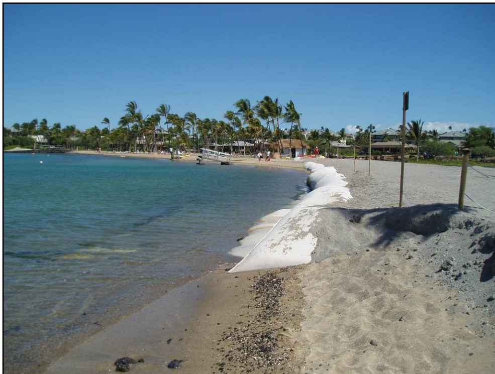
Figure 1-7 Temporary Repairs in the Tsunami Breach at Waikoloa Beach, as Photographed 20 September, 2011
