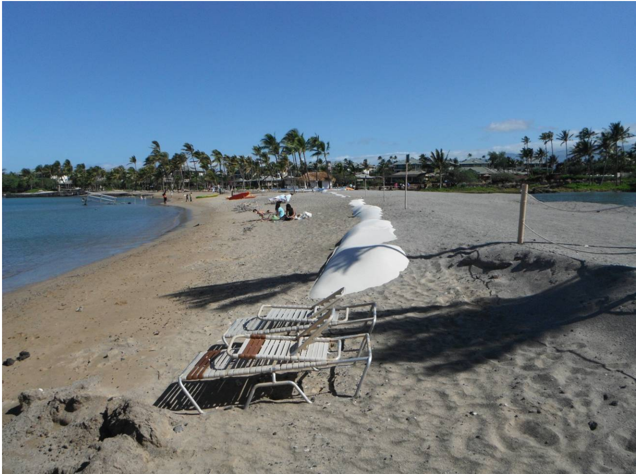
Figure 1-9 Temporary Repairs in the Tsunami Breach at Waikoloa Beach, as Photographed 14 March, 2012
