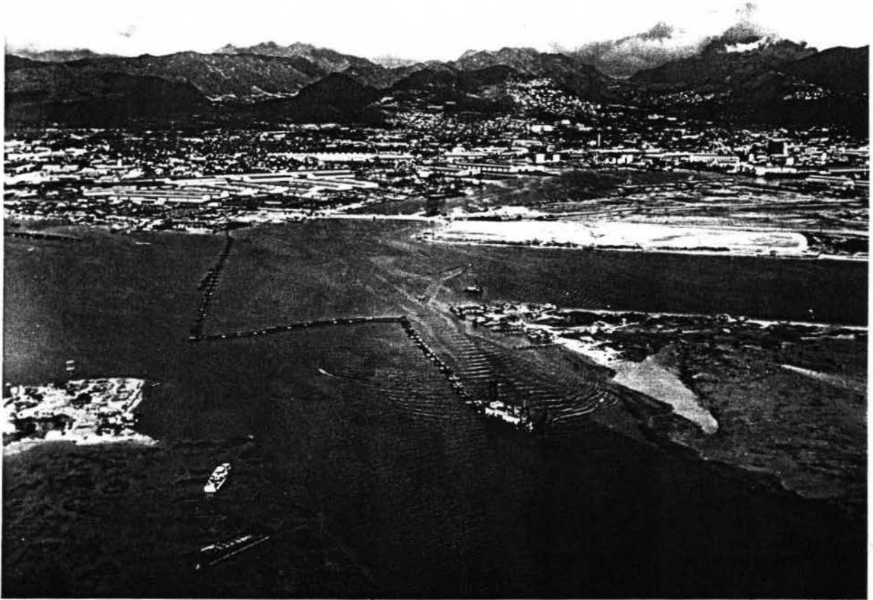
Dredging of Honolulu, 2nd Entrance Channel by Hawaiian Dredging & Co. January 1960. Shows residences on Mokauea Island as well as Harris which was formed by dredging spoils. USCE photograph #687.
