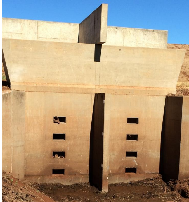
Figure 1: Honokawai reservoir drainage port openings. Sixteen design scenarios considered combinations of closing and modifying the openings of the reservoir to alter the drainage times, and the sediment retention, in Honokowai #8 reservoir. Evidence of recent sediment removal in front of the ports is seen in this photo from September 2014.
