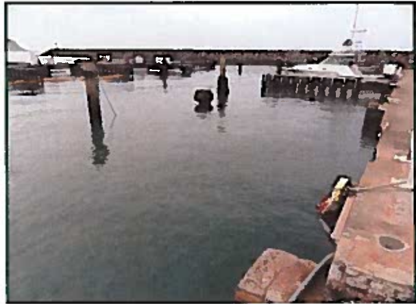
View of Pier B with cracked and missing catwalks.
