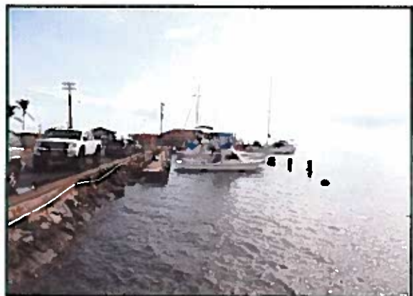
Tahiti moorings at Kaunakakai Pier.
