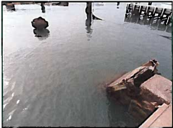
Fallen catwalk on Pier B.
