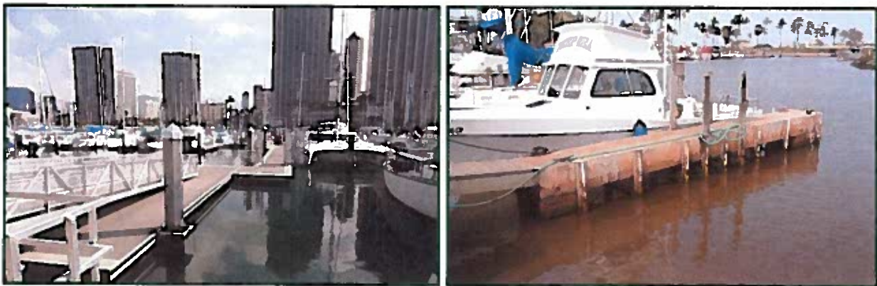
Representative floating catwalk at Ala Wai small boat harbor made of composite material secured to concrete piles (left photo) and a representative fixed catwalk of wood and concrete construction at Haleiwa small boat harbor (right photo).
