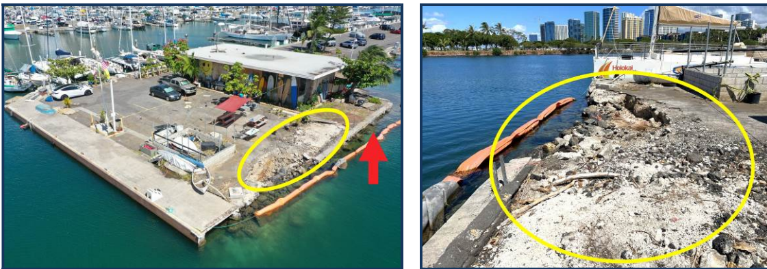
Approximate location of the further detached portion of the makai pier (additional 600 SF) annotated in red arrow. Approximate location of the sunken-in portion of the fast land annotated in yellow outline (approx. 700 SF).
