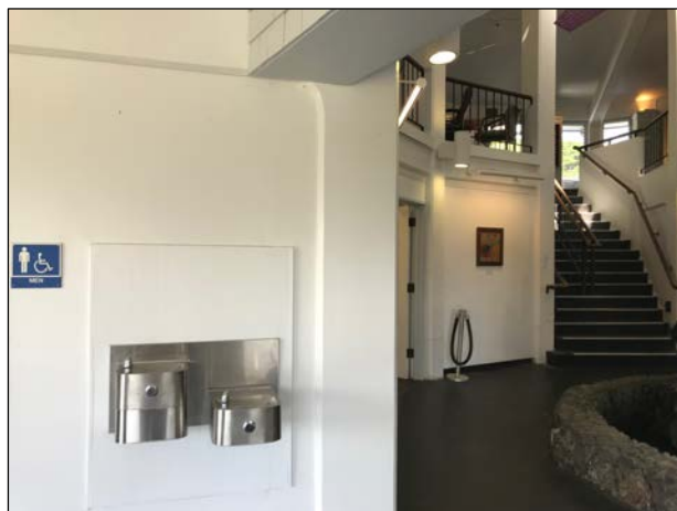
Wall-mounted water fountain within the Center building.
