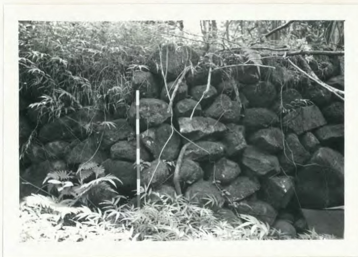
Figure 9. Portion of an agricultural terrace, showing detail of construction. Photo taken facing south (upslope).
