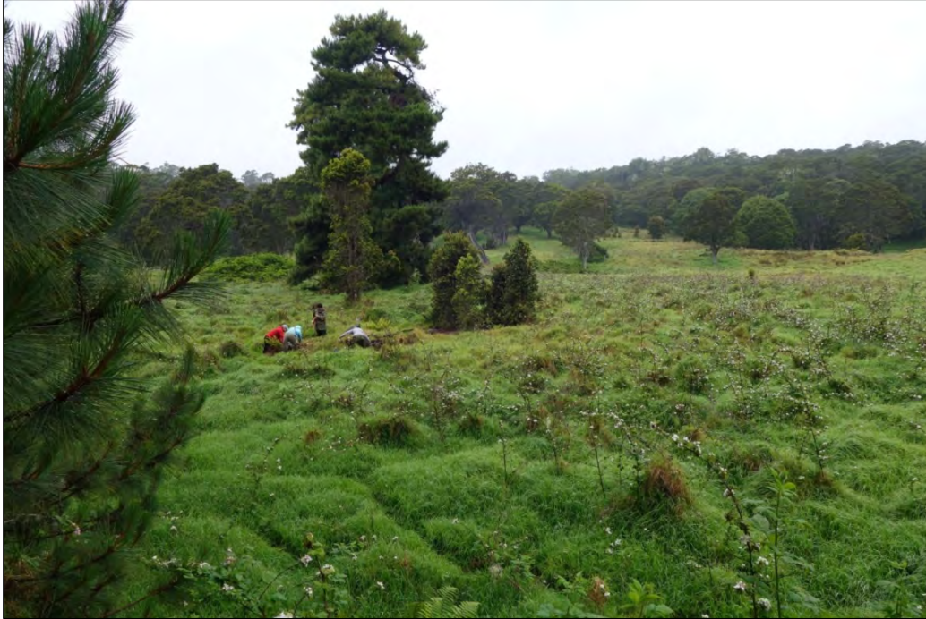
Figure 33: Inspection Team Recording Collapsed Remains of the Shelter and Water Tank (View Facing West). Note the mix of blackberry bushes amongst the kikuyu grass hummocks.
