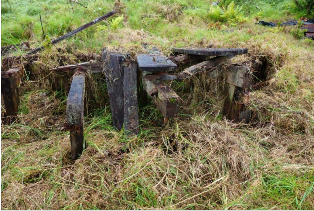
Figure 31: Foundations of the Shack Camp Water Tank Located Adjacent to the Shelter.
