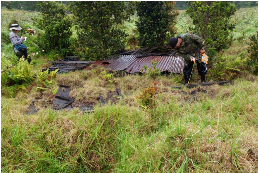
Figure 30: Collapsed Structure of the Shack Camp Shack (View Facing West). The layout and construction of the shack is still recognizable, including the corrugated iron roofing, wooden board and batten walls, nails, and door.
