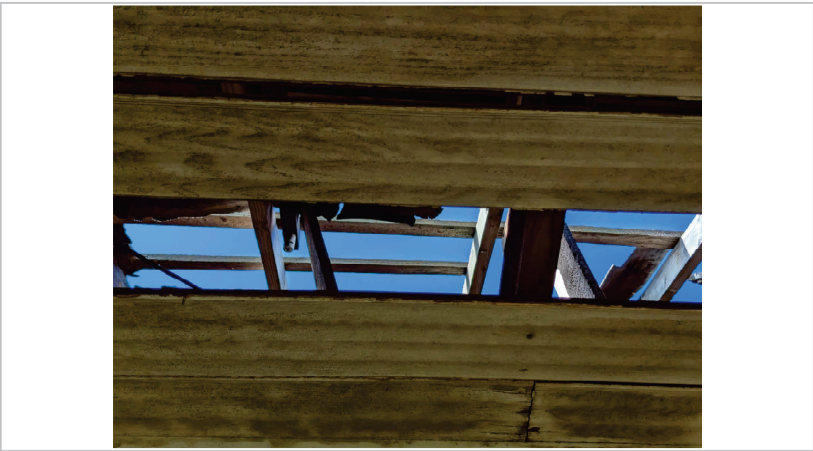
Image Description: Close up of Broken Roof
