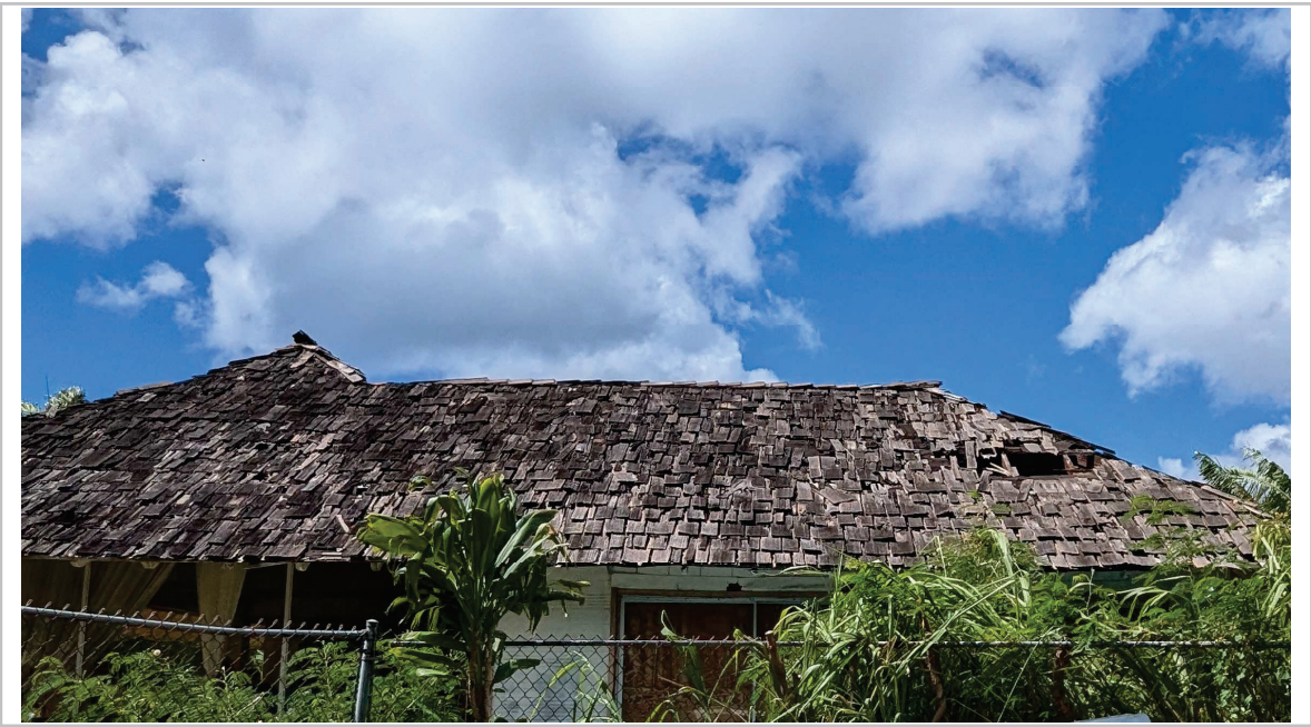
Image Description: Roof to be replaced
