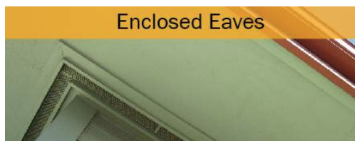
Figure 36. Make sure your eaves are enclosed with non-combustible materials to prevent ember entry.
