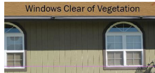
Figure 10. Keep windows free of vegetation to reduce likelihood of heat-caused breakage that lets embers into your home.
