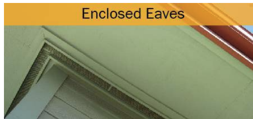
Figure 11. Make sure your eaves are enclosed with non-combustible materials to prevent ember entry.
