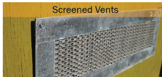
Figure 12. Covering vents with 1/8-inch or smaller metal mesh blocks embers from entering a home or structure.
