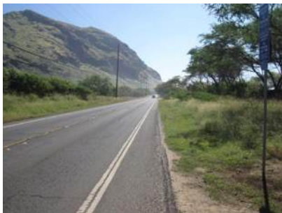
Highway along Kea'au Beach Park with no drivable shoulders
