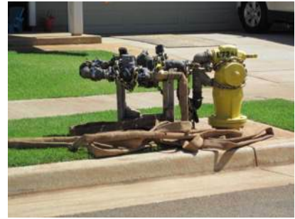
Fire hydrant and hose on Kekahili Street
