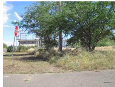
Electric facility surrounded by kiawe and grass along FDR Avenue
