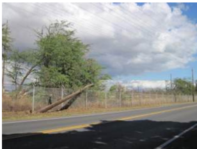
Downed utility pole next to wildland area along FDR Avenue
