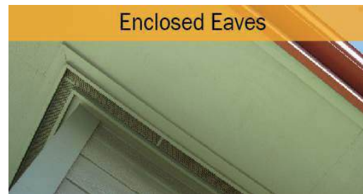
Figure 14. Make sure your eaves are enclosed with non-combustible materials to prevent ember entry.
