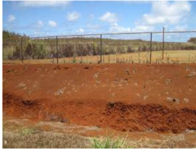
King Kaumuali'i Elementary School with eroding slope
