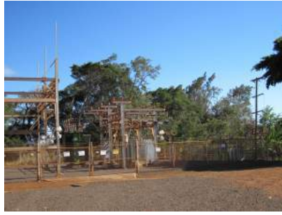
Overgrown fuels next to power generator
