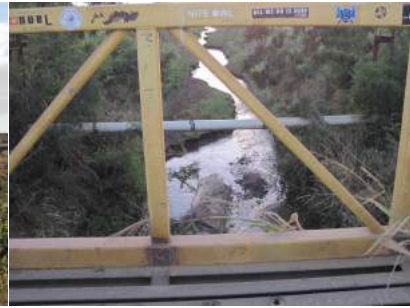
Stream with heavy erosion and fuel-build-up on road to Polihale
