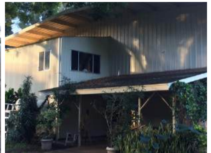
Seabury Hall, example of debris on roof
