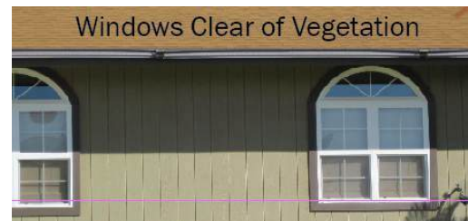
Figure 13. Keep windows free of vegetation to reduce likelihood of heat-caused breakage that lets embers into your home.
