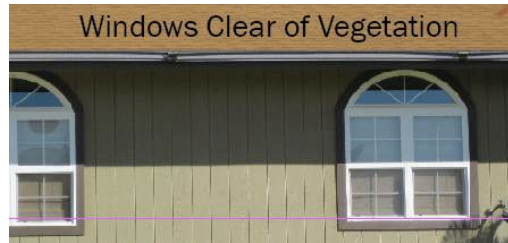
Figure 35. Keep windows free of vegetation to reduce likelihood of heat-caused breakage that lets embers into your home.
