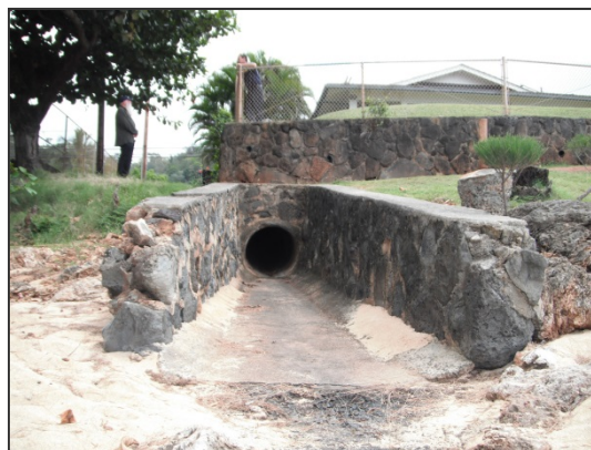
This storm drain runs beneath the fire station and drains the Foodland parking lot.
