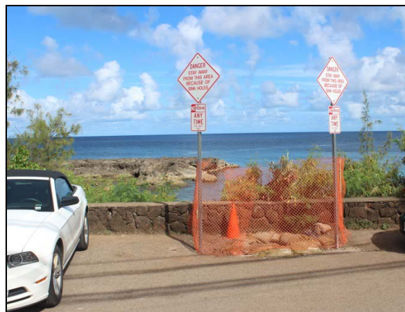
Portions of the rock wall are being undermined by erosion.
