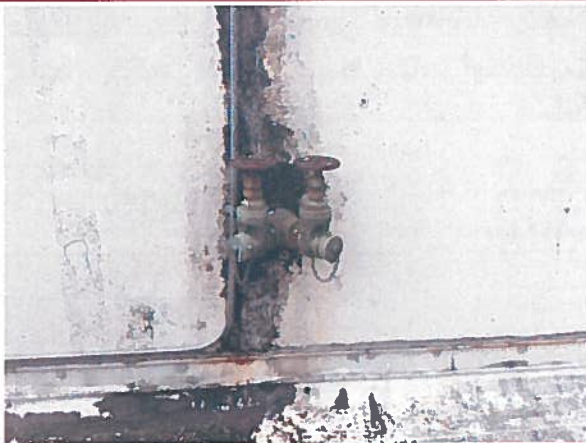
Please ensure all Fire Department Connections are in working order, as many are not in operational order at this time
