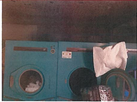
Ensure that laundry equipment is properly installed and has adequate venting, as ceiling shows signs of heat damage
