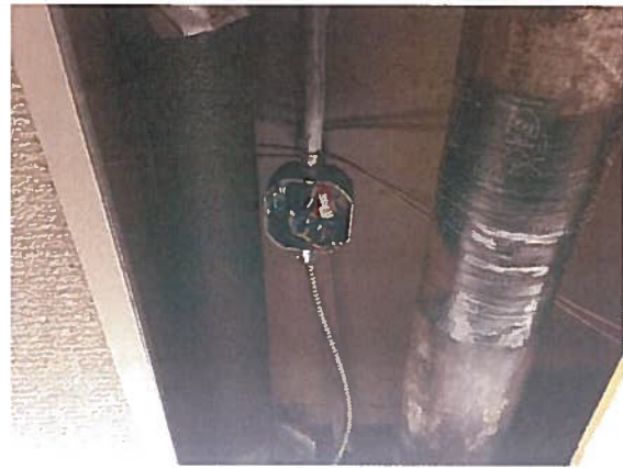
Junction boxes need to be covered to assist in Fire Prevention
