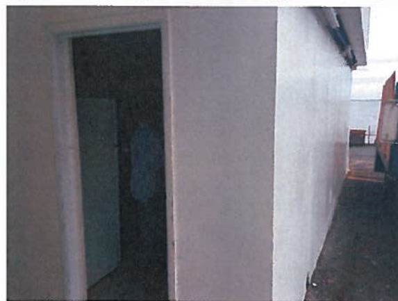
Storage on bottom has non Fire rated door, which may not be able to protect room and contents
