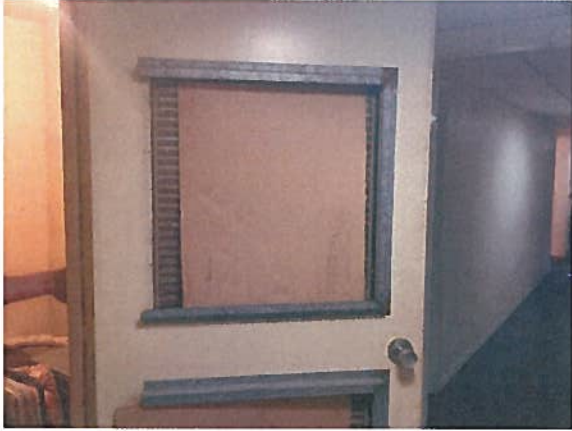
Remove cardboard from rated fire doors
