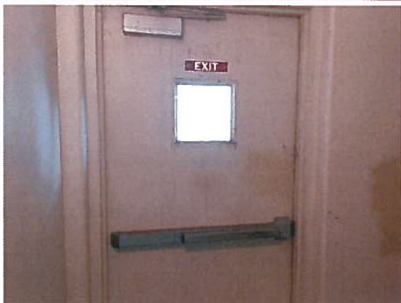
The door on the ground floor facing the ocean in rear stairwell needs to be fully operational. *DOOR HAS BEEN INTENTIONALLY DISABLED*
