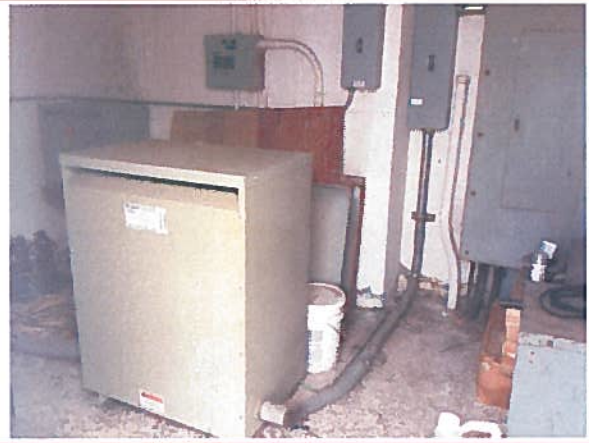
Please remove combustible storage from transformer room
