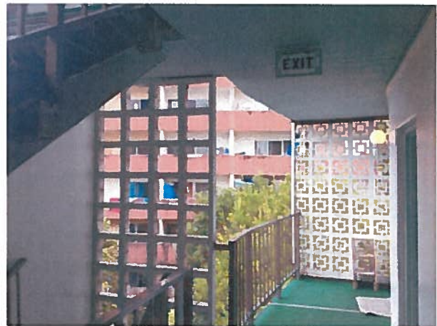
Please ensure exit signs are in proper working order
