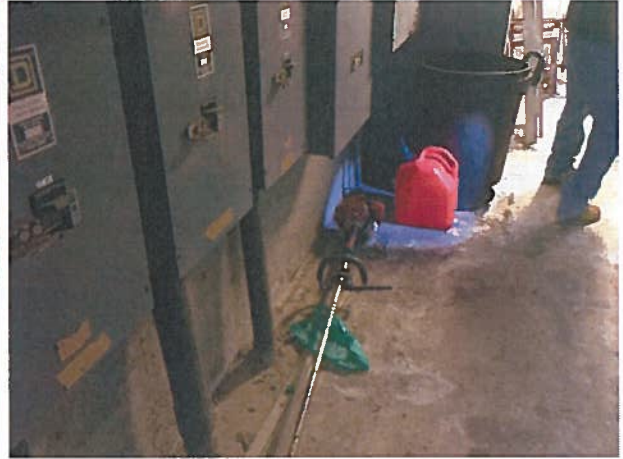
Remove combustible liquid and related equipment from main electrical room
