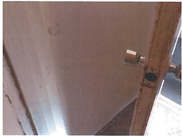
All hardware for doors shall be working and in good operational condition
