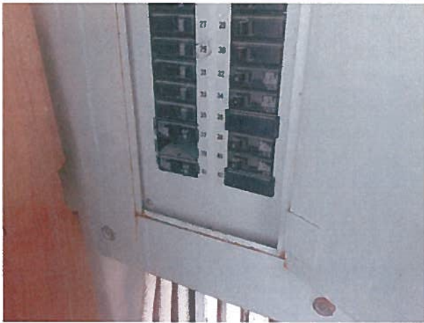
Electrical panels need to have open circuits covered
