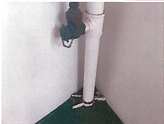
Please ensure Fire Department Standpipes are properly secured, as bracing has not been maintained
