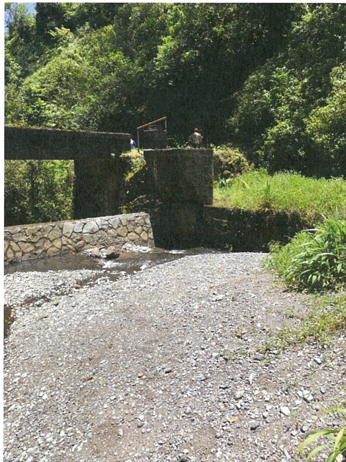
Figure 11. Dam, gate, and control structure at K-21.
