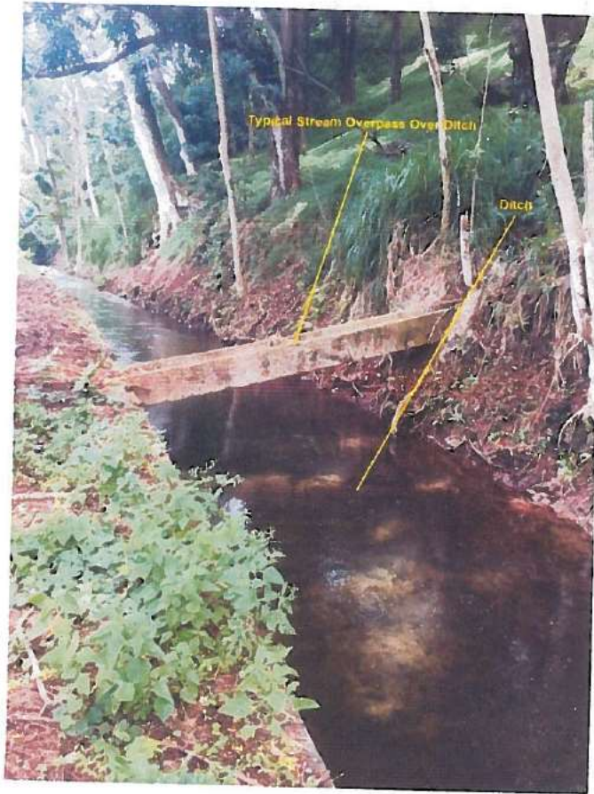
Photo 14 (above): Typical “stream overpass” intended to prevent the ditch from intercepting a stream
