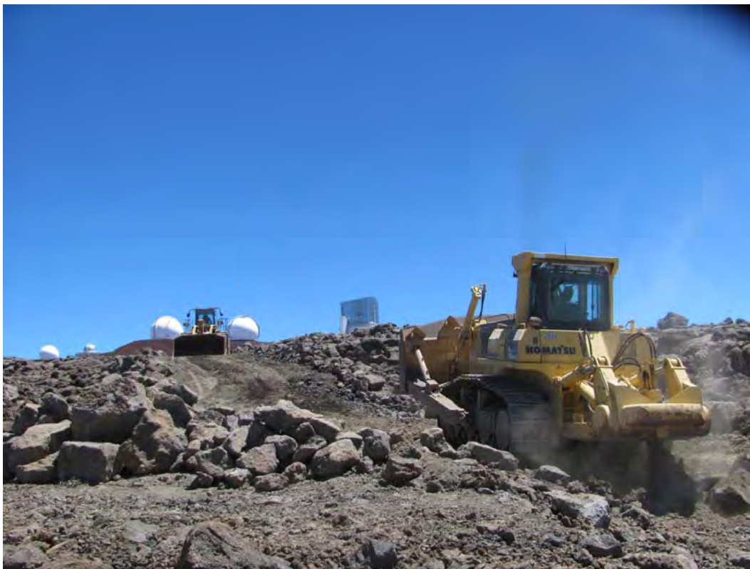
Figure 7. Komatsu 275AX bulldozer and Komatsu WA500 loader grading the existing 4WD road, note observatories in background.
