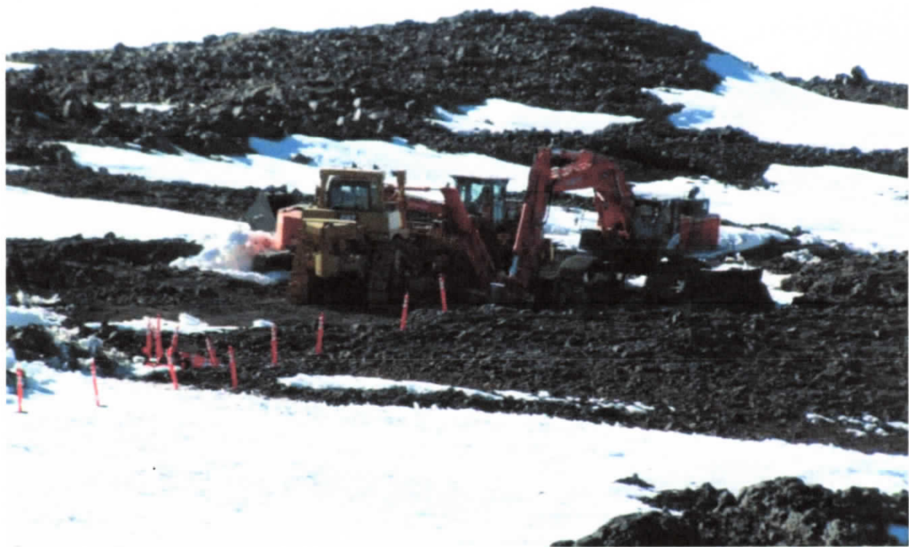
Heavy construction equipment used for groundwork, excavation, and grading during geotechnical boring in August-October 2013 at the proposed TMT site on Mauna Kea.
