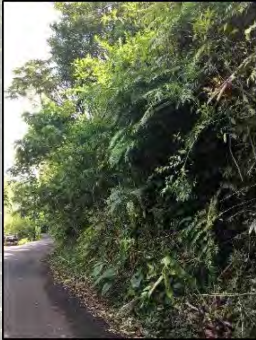
Vegetation Encroaching on Roadway
