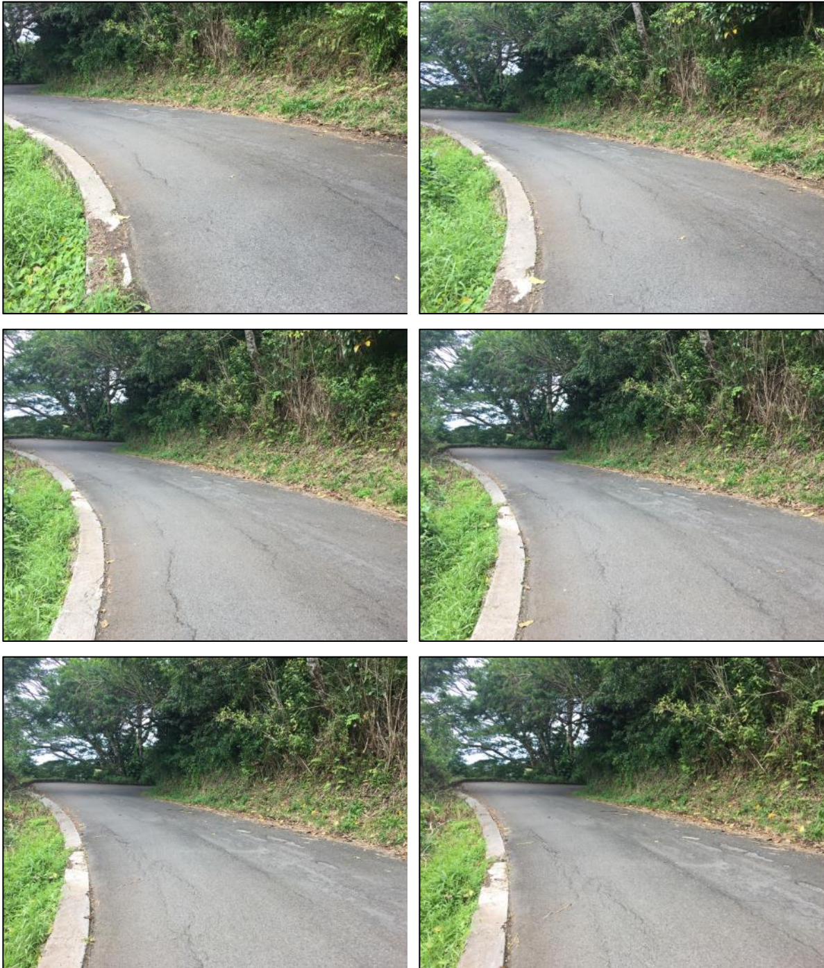
Figure 3.9 Subsidence between 3811 Tantalus Drive and Pu‘u ‘Ōhi‘a Trailhead
