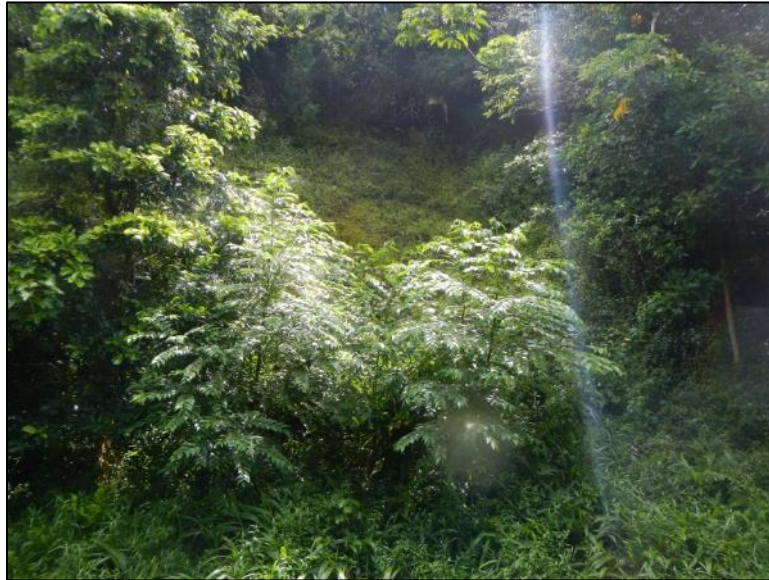
Figure 3.16 Embankment Issues between 3811 Tantalus Drive and Pu‘u ‘Ōhi‘a Trailhead
