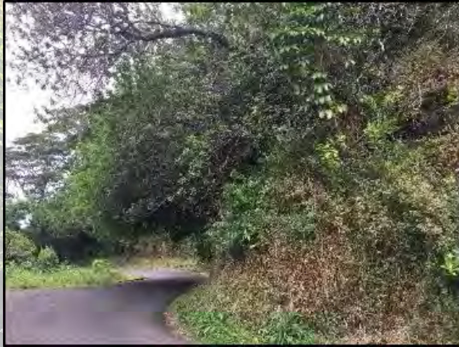
Overhanging Vegetation Restricting Vertical Clearance
