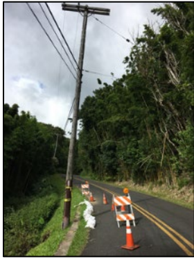
Figure 3.15 Embankment Issues above Forest Ridge Way
