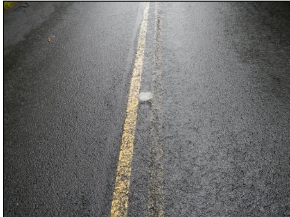
Reflector missing from roadway centerline.
