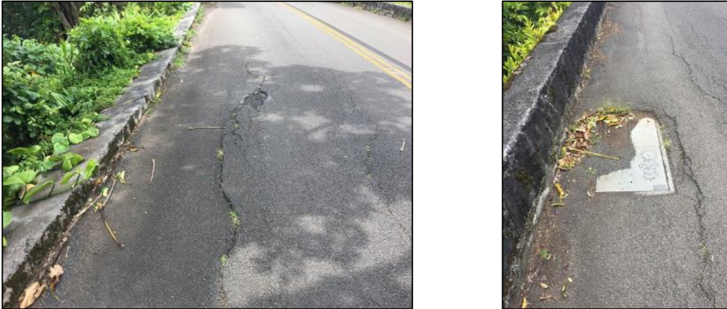
Figure 3.10 Subsidence on the Hogsback
