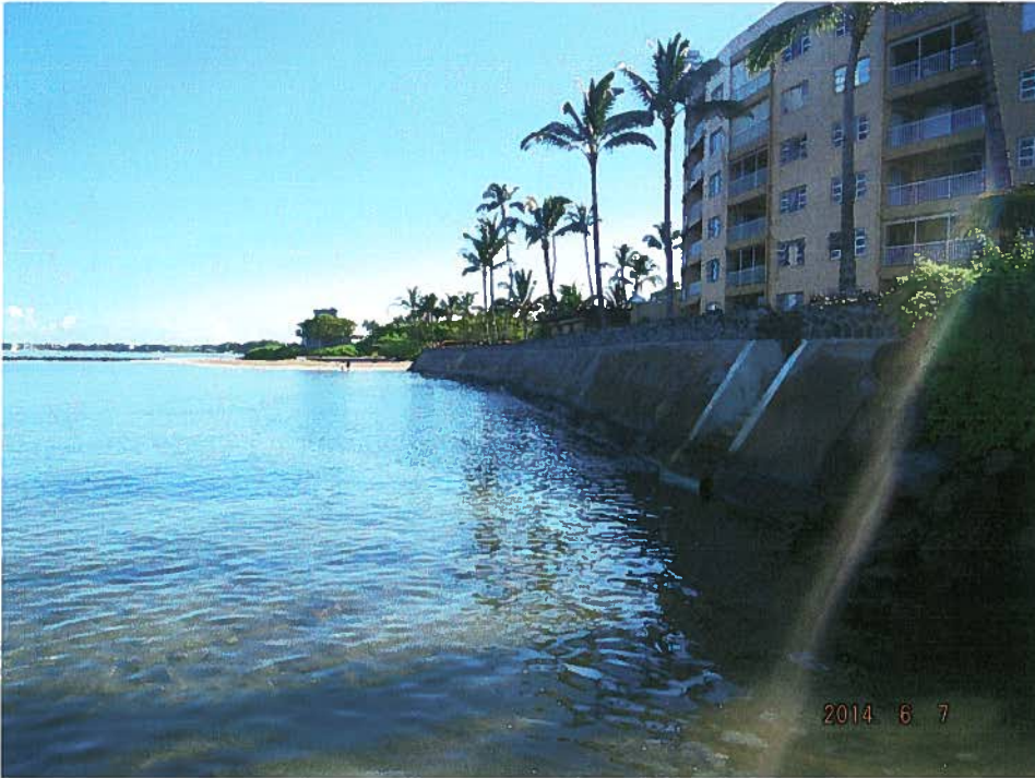
Figure 12. June 7, 2014 Shallow depth at Menehune Shores seawall.
