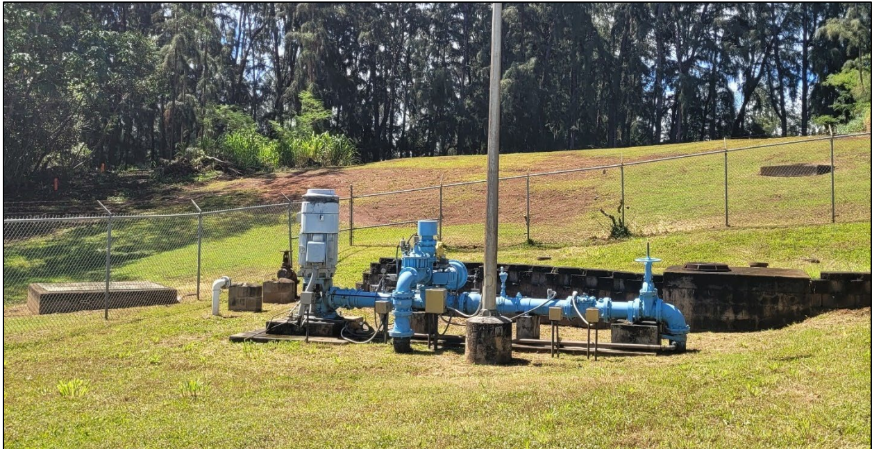
Figure 8: Example of a Similar Production Well
