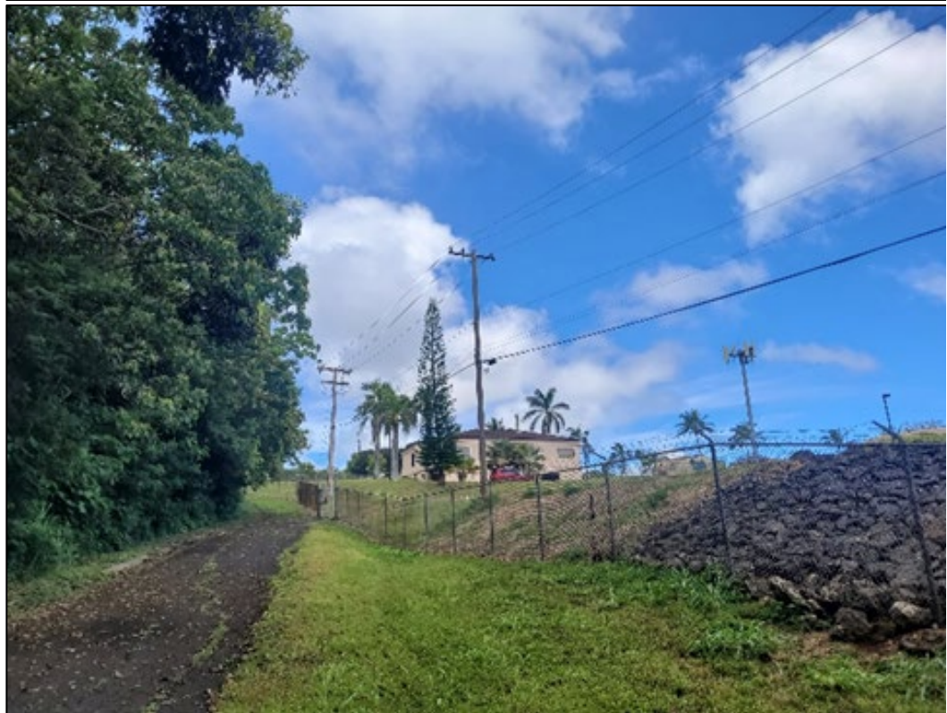
f. View of existing Hawaiian Electric power lines and poles in vicinity of proposed tap.
