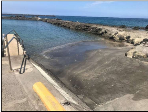
(a) May 2018. Concrete boat ramp with accreted sand.
