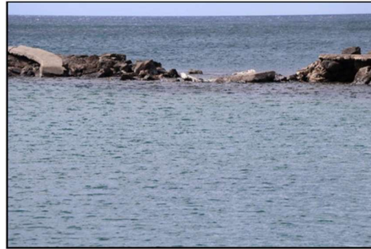
(b) January 2020. Breached section of Main Breakwater.
