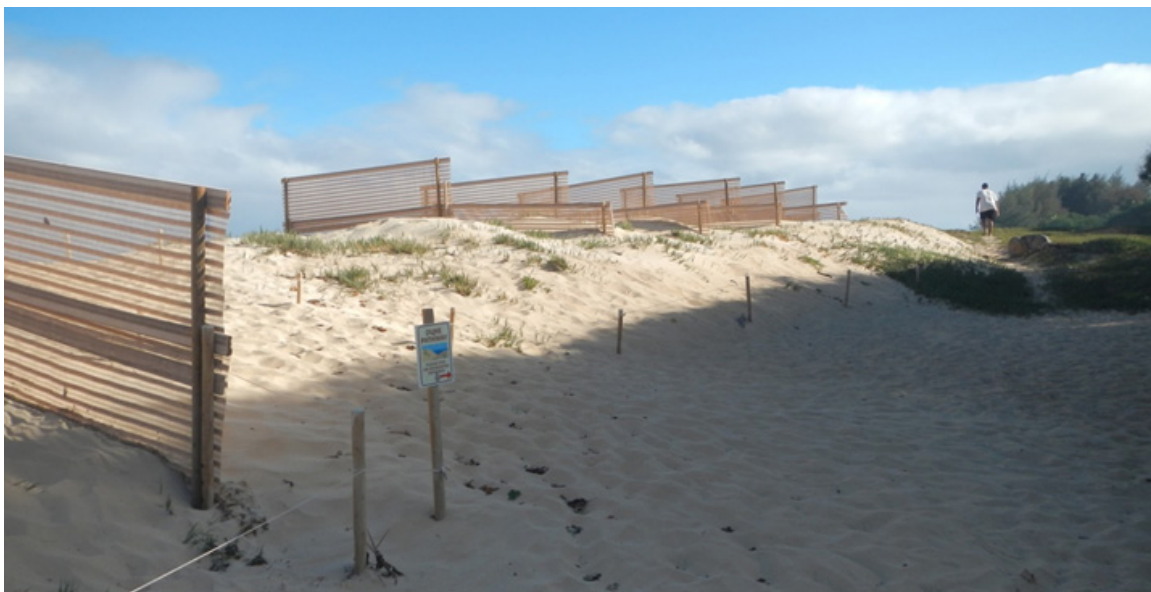
FIGURE 26. Sand fencing was installed at Kanahā Beach Park on the north shore of Maui to capture wind-blown sand and stabilize restored dunes. Sand fence panels eventually require maintenance or removal.
