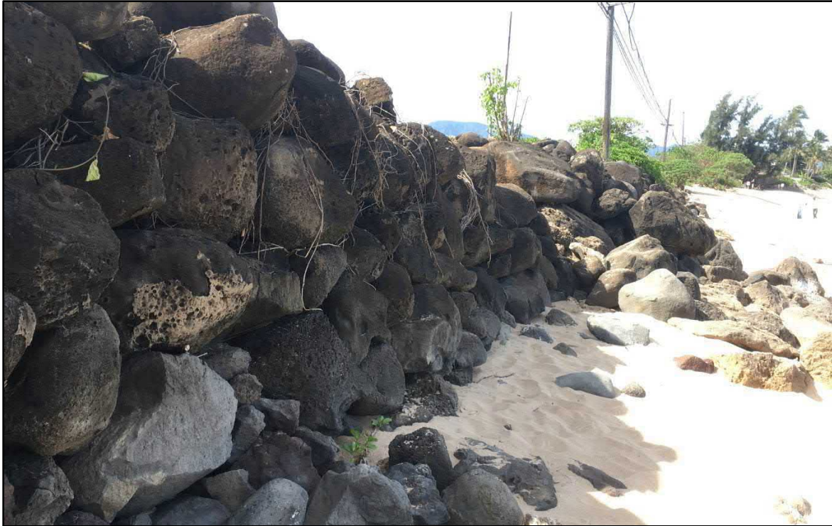
Figure 2-15. Revetment reach shown original wall structure (foreground) and damaged area
