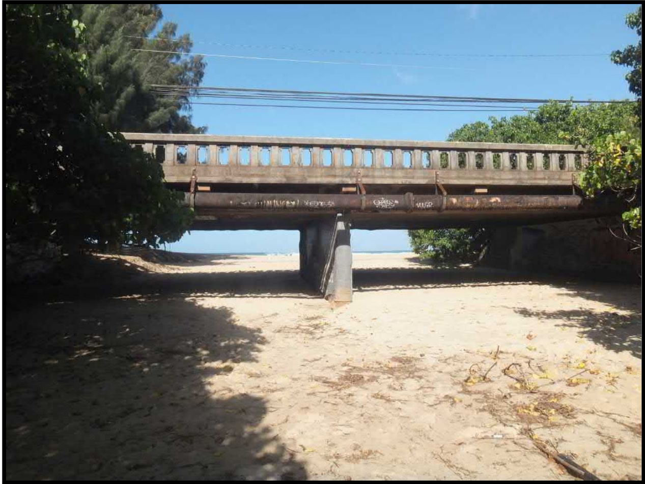
Figure 3-9. Existing Bridge Over Lauhulu Stream (Also Referred to as Laniakea Stream or Kukaiohiki Gulch)
