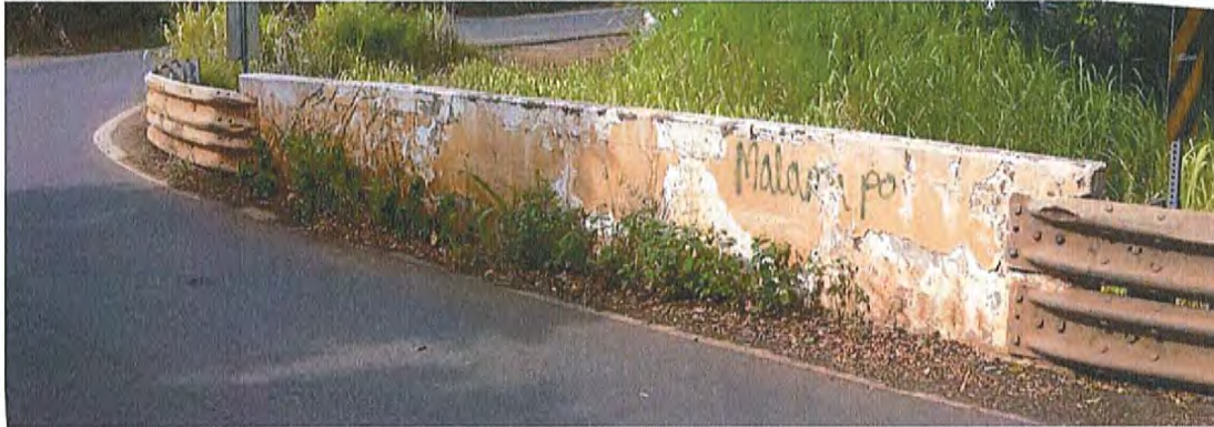
Photograph 5. HI_MauCounty_HonoluaStreamBridge_0005. Parapet on the downstream side of the bridge. Note the repaired section at the far end. View facing southwest.
