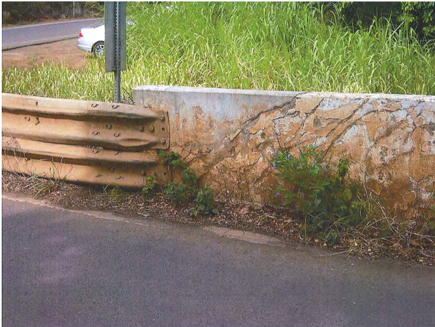
Photograph 9. HI_MauiCounty_HonoluaStreamBridge_0009. Detail of the repaired area of the downstream parapet. View facing southwest.
