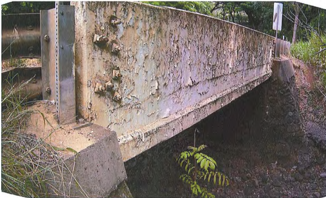
Photograph 7. HI_MauiCounty_HonoluaStreamBridge_0007. Outboard side of the upstream parapet. Note the beveled string course at the lower edge of the parapet. View facing northwest.
