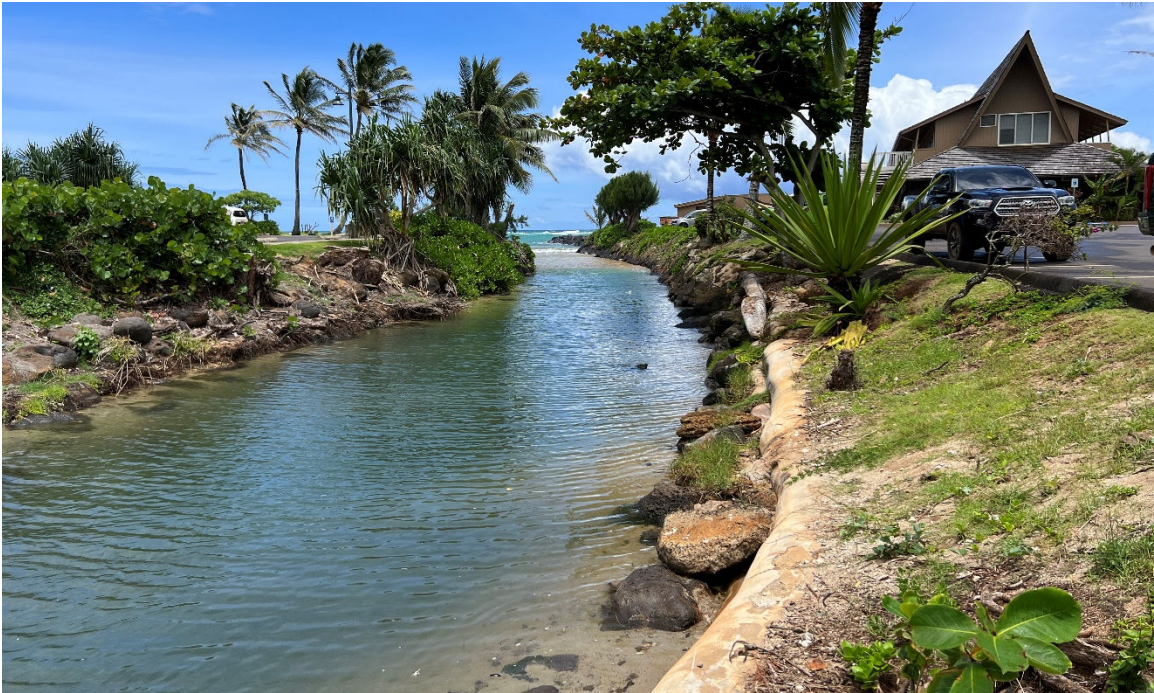
Figure 12. Photograph taken during construction, on May 17, 2023, showing the dredged Waipouli Drainage Canal, facing east
