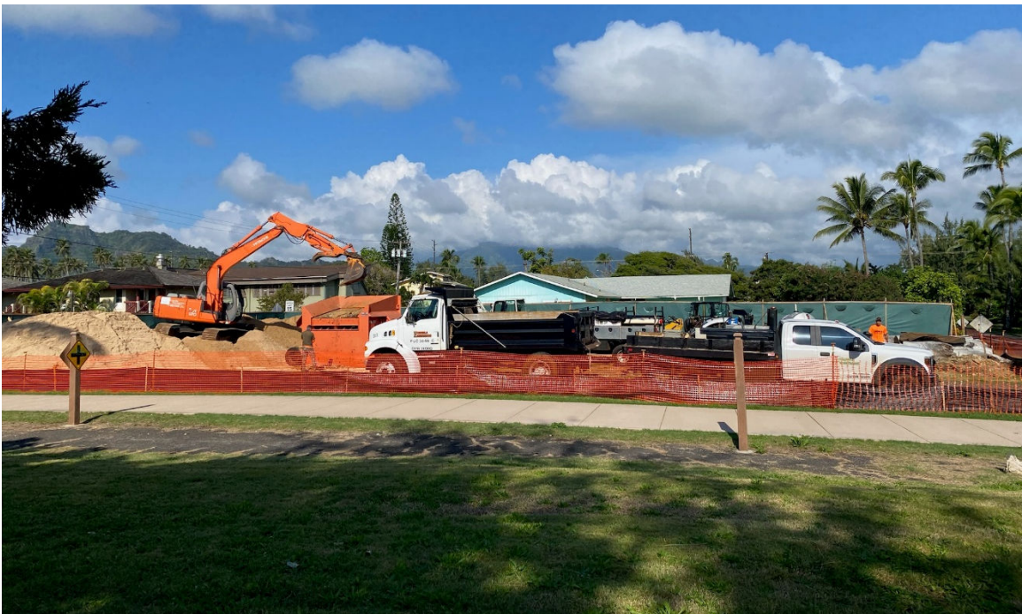
Figure 8. Photograph taken during construction, on February 8, 2023, showing temporary sand stockpiles being screened for coral fragments, with geotextile foundation fabric, fiber roll and silt fence BMPs
