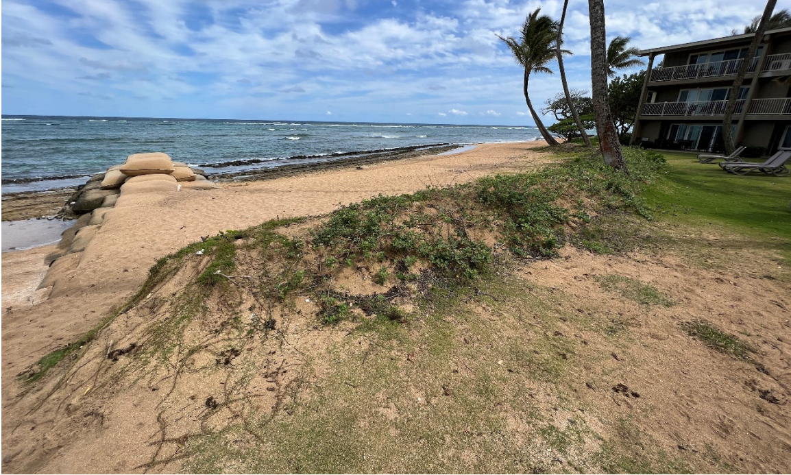
Figure 15. Photograph taken after vegetation establishment, on March 19, 2024, showing sandbag groin, beach nourishment and vegetated sand berm, facing south
