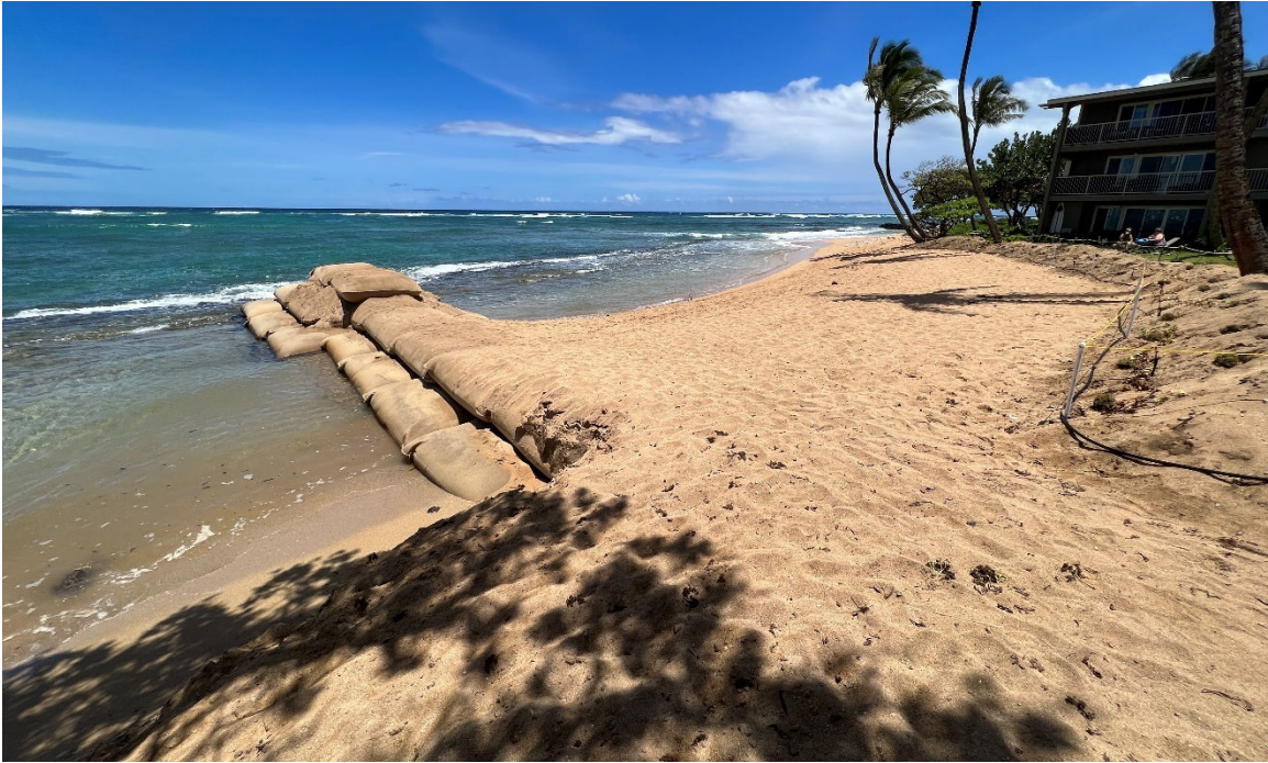
Figure 13. Photograph taken during construction, on May 17, 2023, showing sandbag groin, beach nourishment and unvegetated sand berm, facing south
