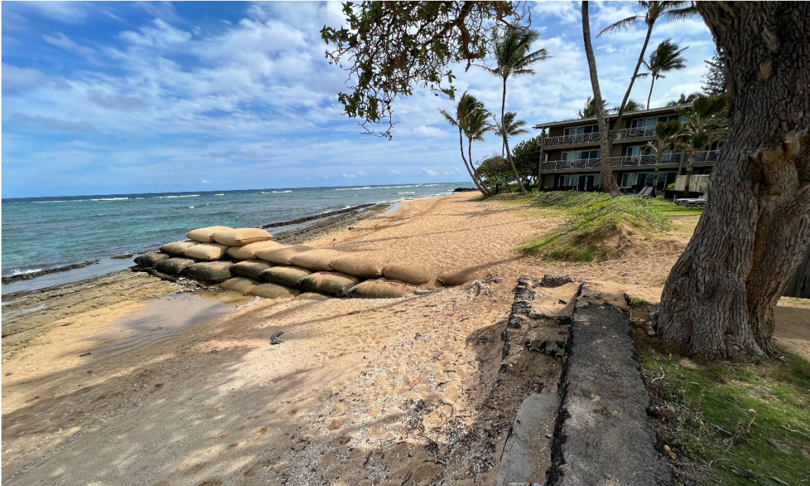
Figure 16. Photograph taken after vegetation establishment, on March 19, 2024, showing sandbag groin and beach nourishment abutting adjacent property to the north, facing south
