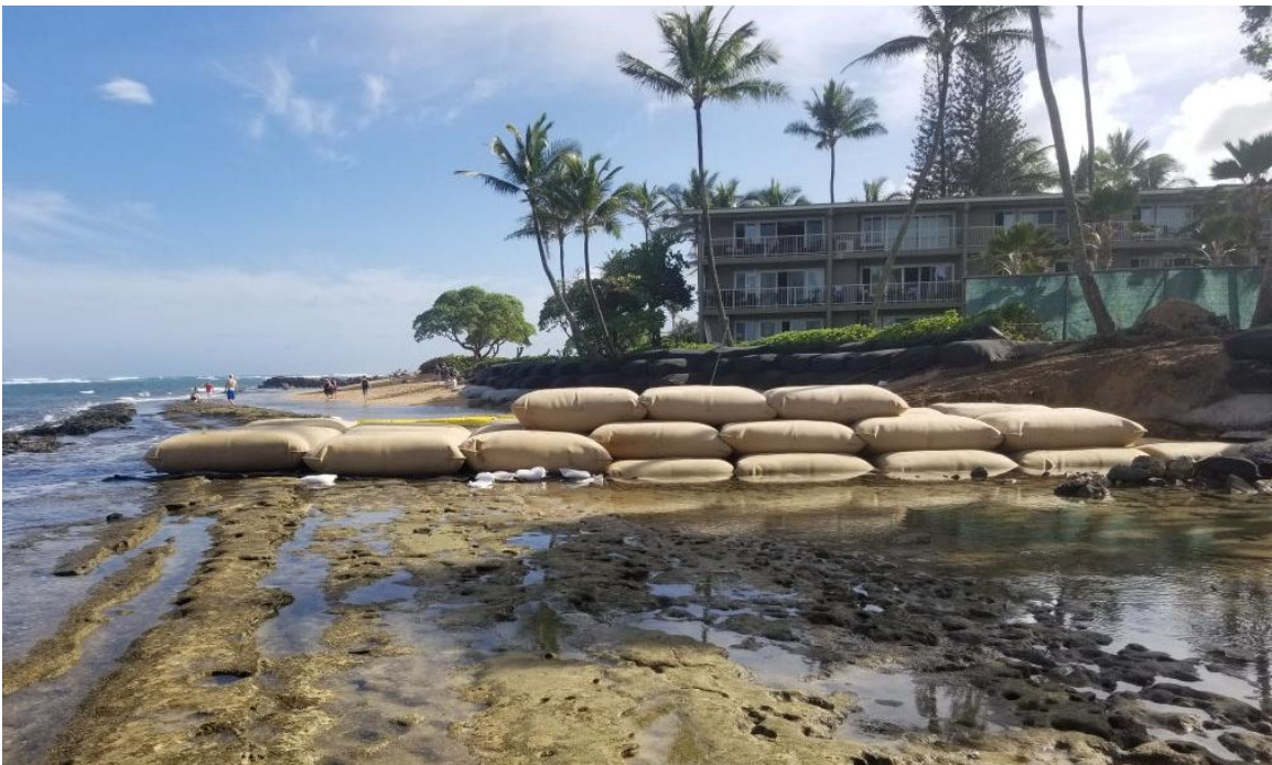
Figure 10. Photograph taken during construction, on March 31, 2023, showing installation of the sandbag groin during low tide, facing south
