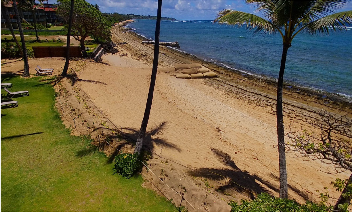
Figure 23. Photograph taken on June 6, 2023, at 12:05 PM, after sand fill and groin placement
