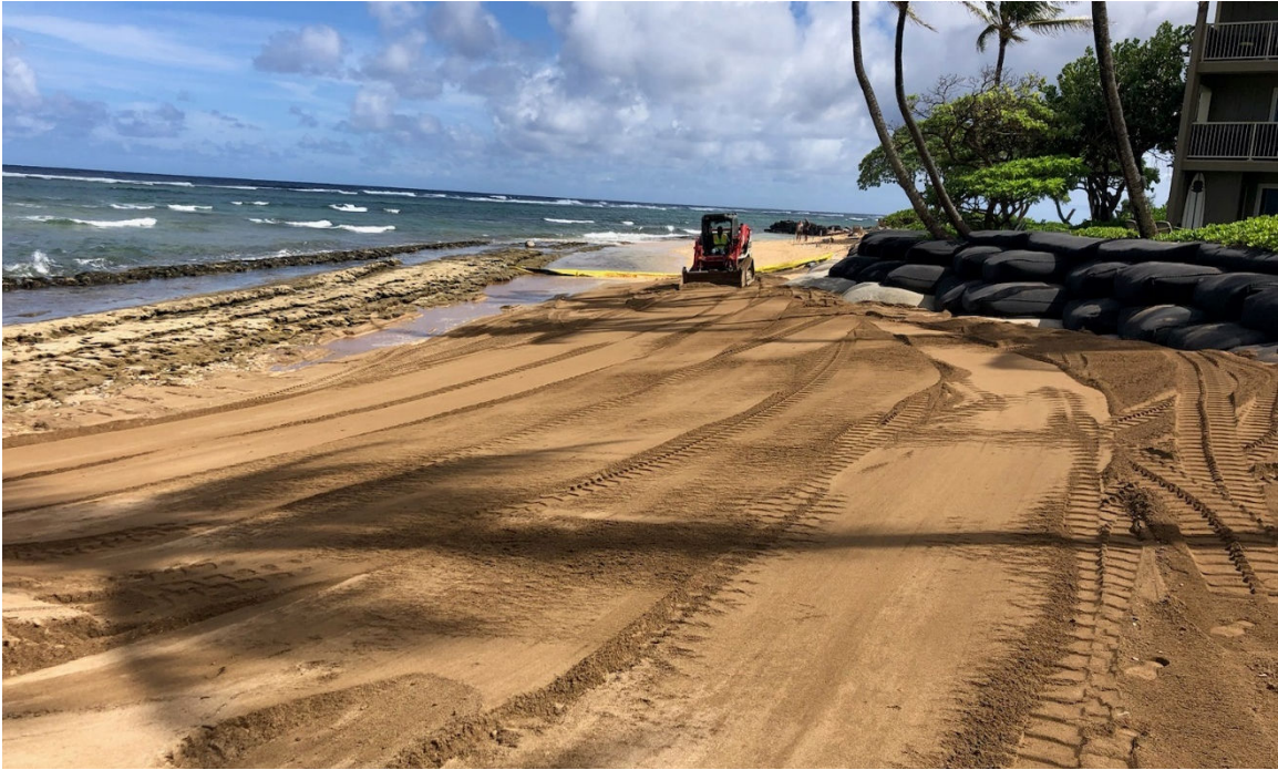
Figure 11. Photograph taken during construction, on April 10, 2023, showing placement of beach nourishment during low tide, with silt curtain BMP in place, facing south
