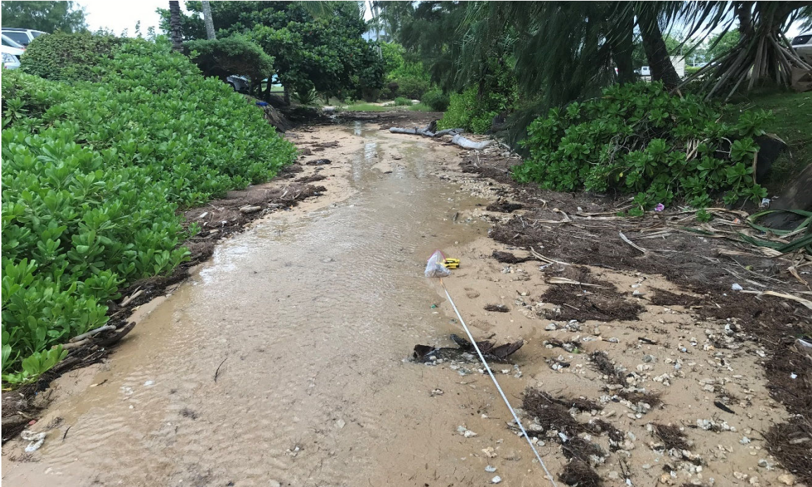
Figure 5. Photograph taken before construction, on August 1, 2018, showing Waipouli Drainage Canal, facing west
