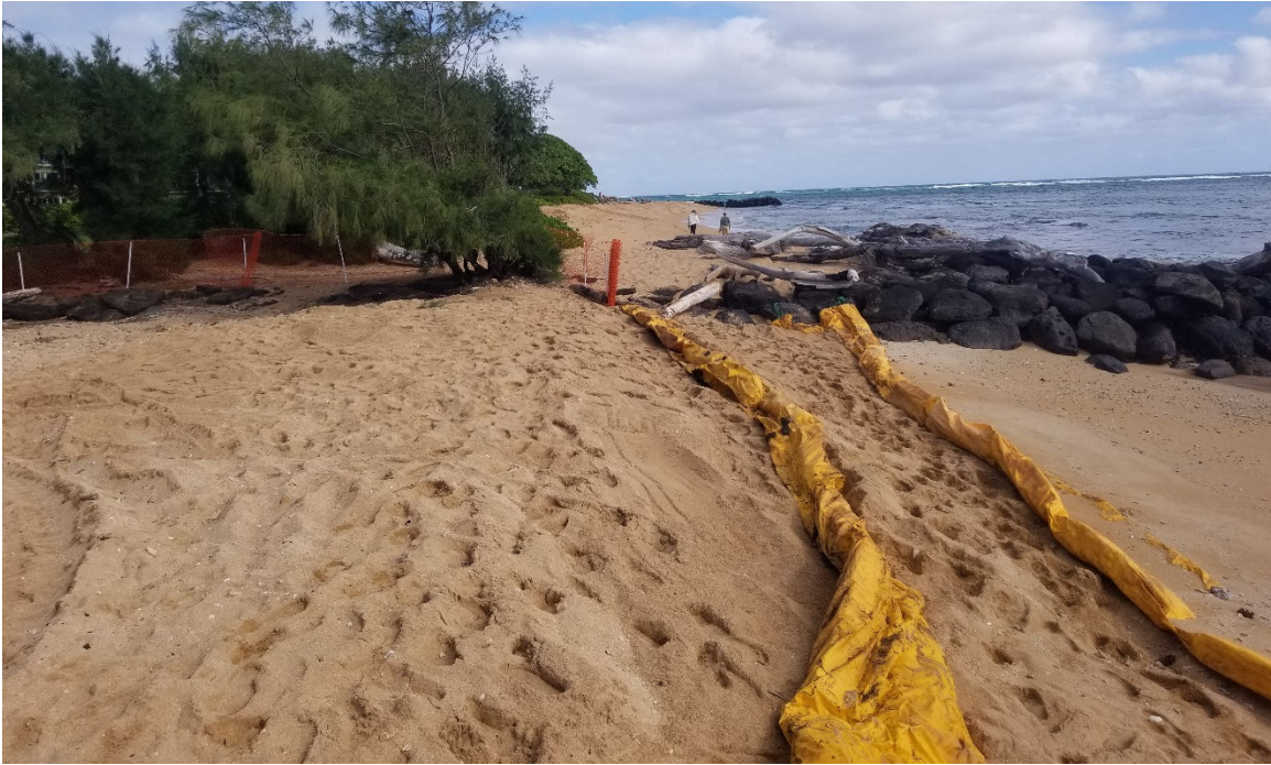
Figure 7. Photograph taken during construction, on February 1, 2023, showing sand plug and silt curtain BMPs at the eastern end of Waipouli Drainage Canal, facing north
