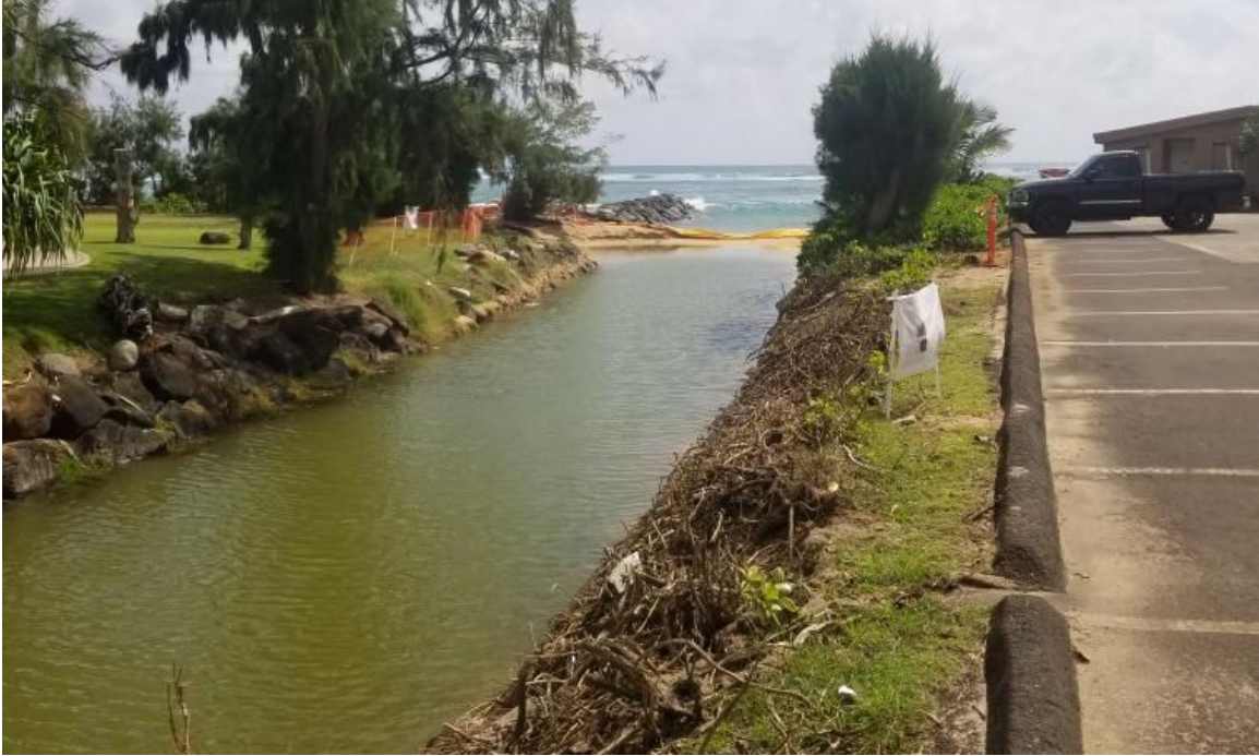
Figure 9. Photograph taken during construction, on February 16, 2023, showing the dredged Waipouli Drainage Canal, facing east
