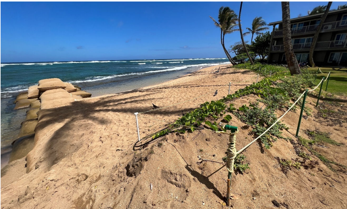
Figure 14. Photograph taken during vegetation establishment, on August 29, 2023, showing sandbag groin, beach nourishment and partially vegetated sand berm, facing south
