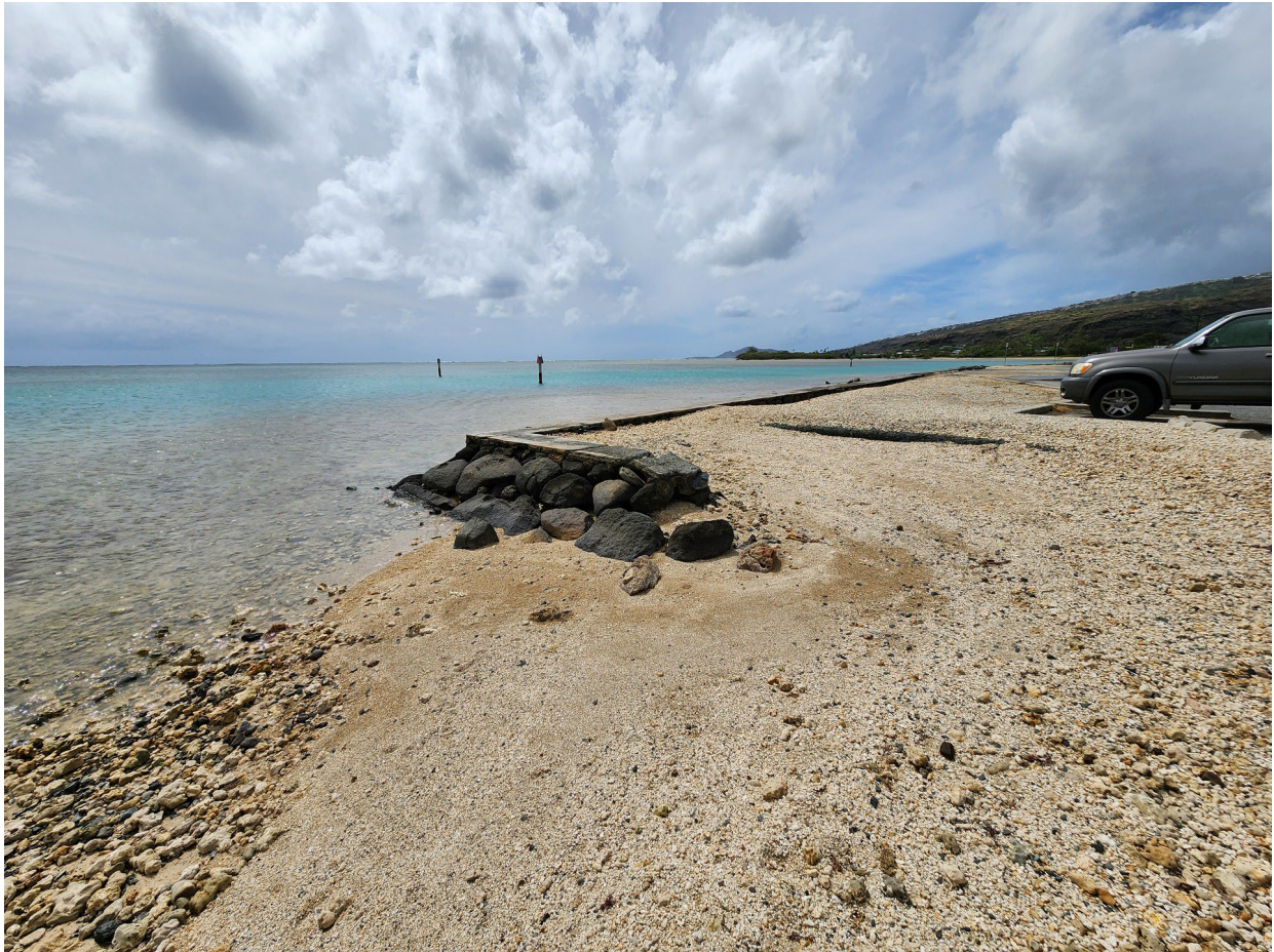
Figure 15. Photo of the Terminal End of the Type B Wall Located at the East End of East Beach.
