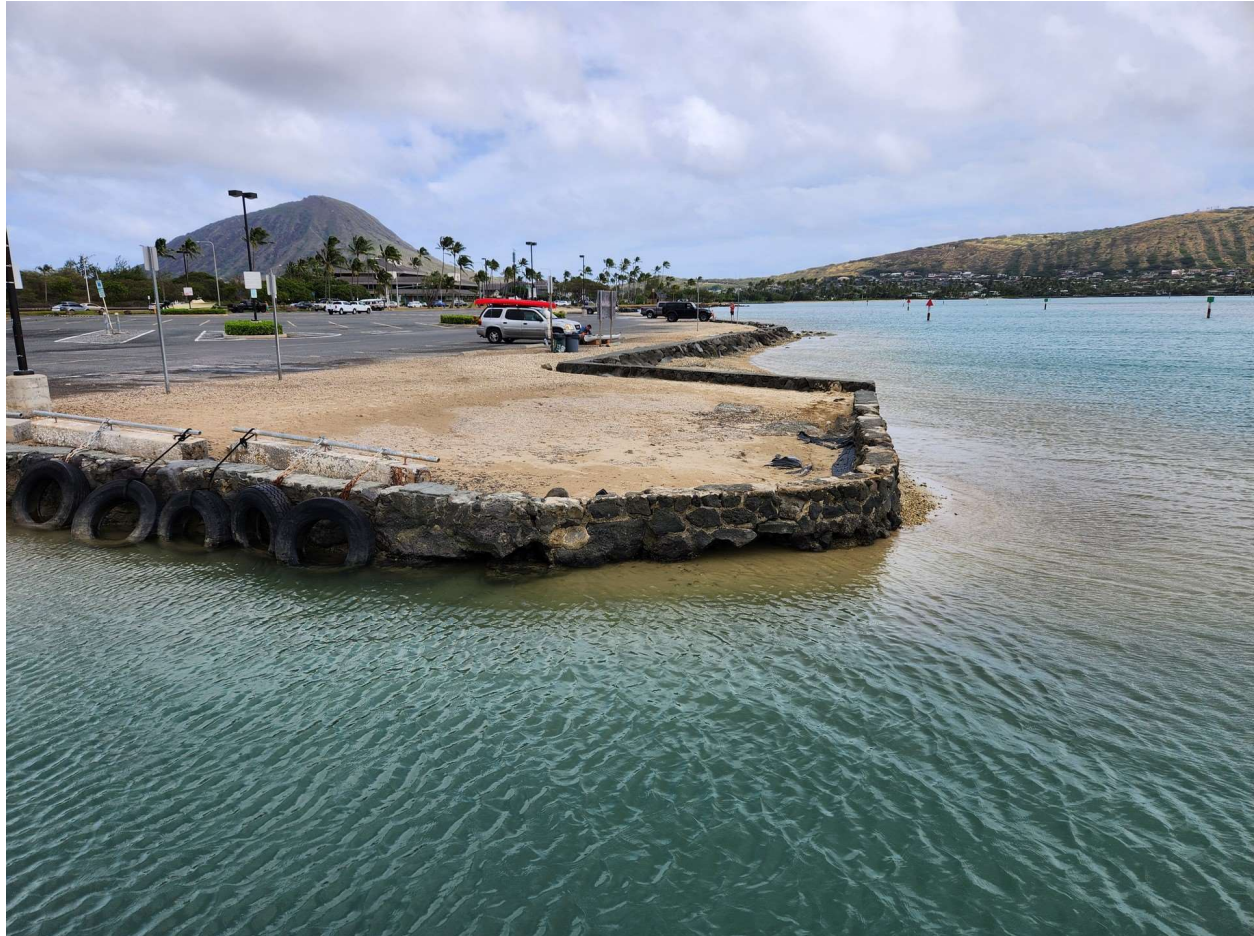
Photograph 7, Photo of the Dilapidated Type A Wall along the East Edge of the Boat Ramp, Looking East, on February 28, 2024 (Photo: Integral Consulting Inc.)
