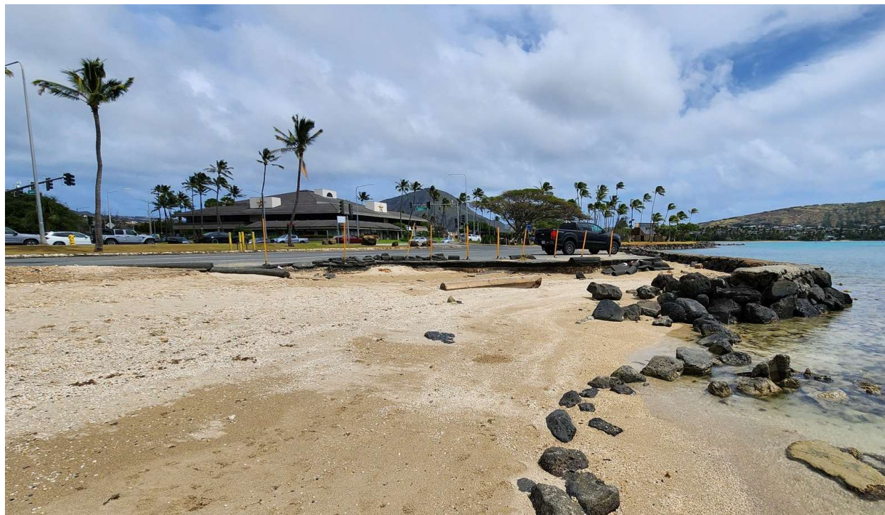
Photograph 9, Photo of the Dilapidated Wall/Revetment Structure and Shoreline Erosion Area Located at the East End of East Beach
