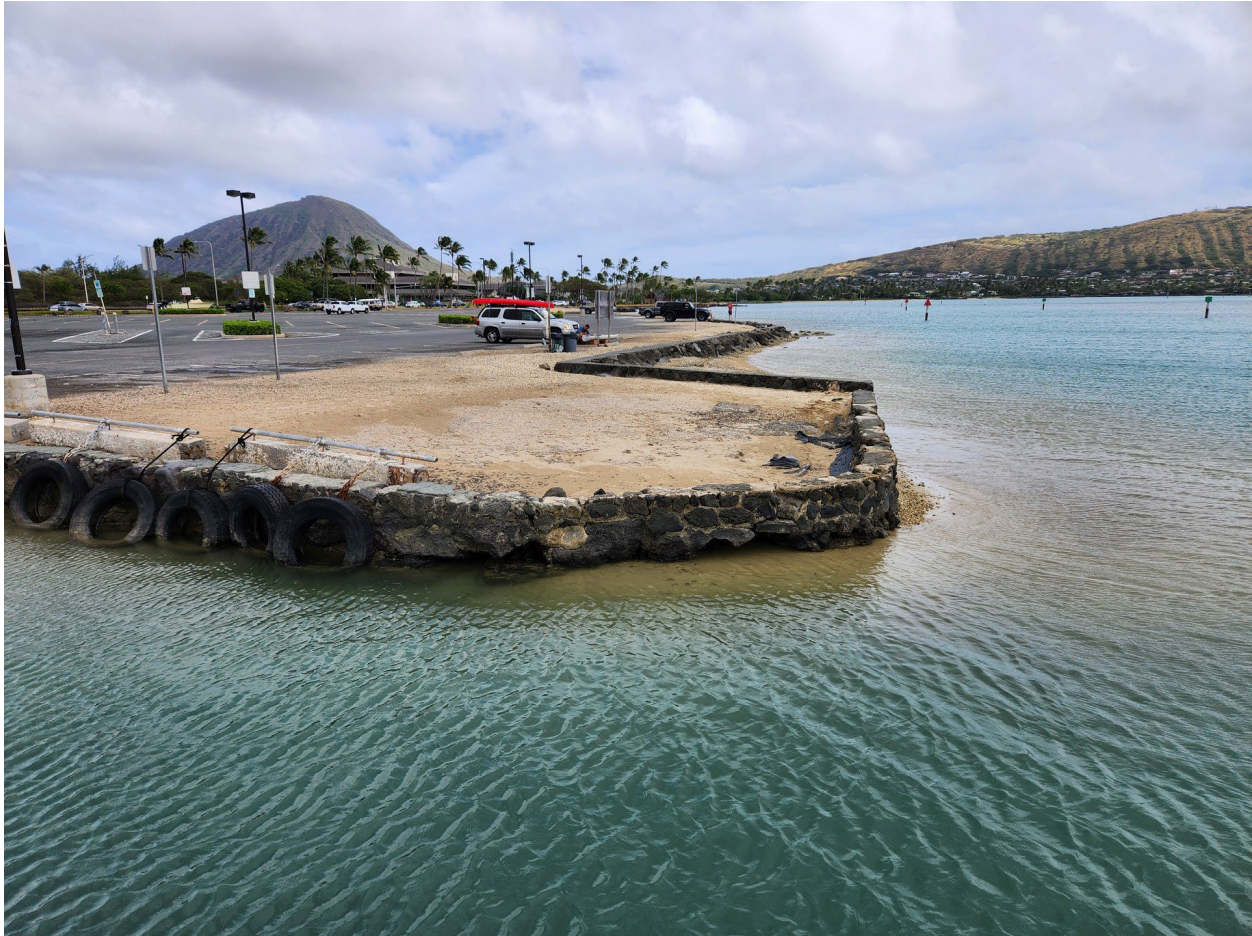
Figure 14. Photo of the Dilapidated Type A Wall along the East Edge of the Boat Ramp, Looking East, on February 28, 2024 (Photo: Integral Consulting Inc.).
