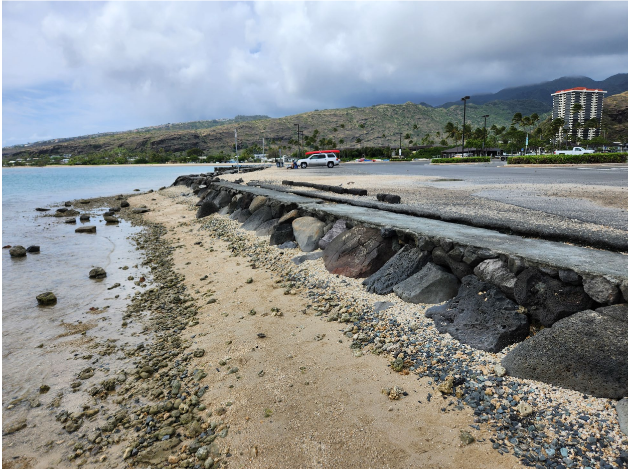
Figure 13. Photo of the Type B Wall East of the Boat Ramp, Looking West, on February 28, 2024 (Photo: Integral Consulting Inc.).
