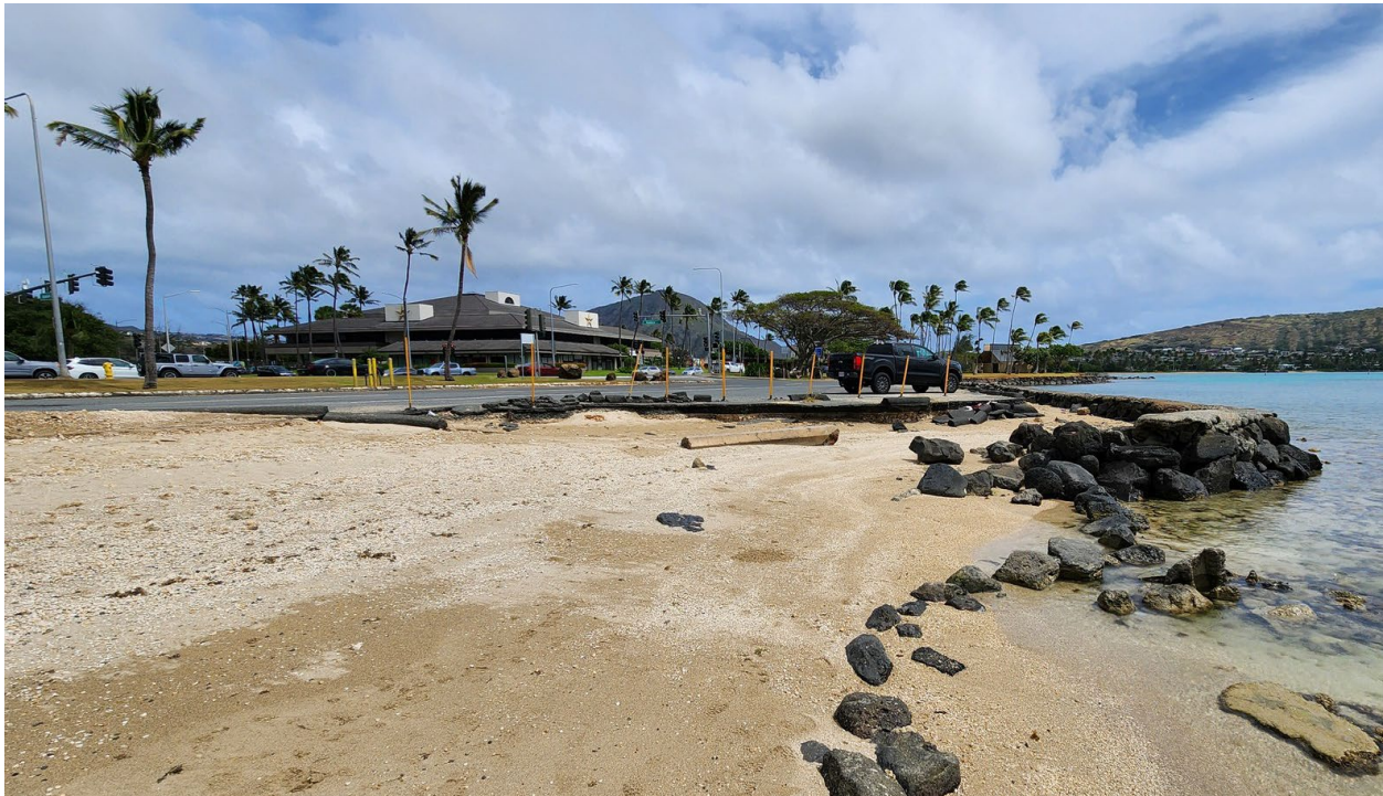
Figure 16. Photo of the Dilapidated Wall/Revetment Structure and Shoreline Erosion Area Located at the East End of East Beach.
