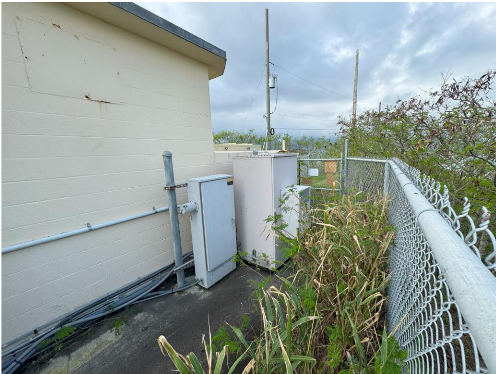
Figure 6: Inside T-Mobile compound View (Existing PPC and BBU).
