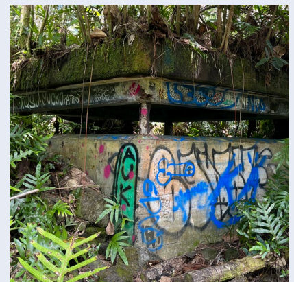
Figure 29. Graffiti on historic WWII bunker along trail
