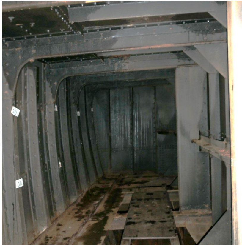
Tank #4 Port, looking forward.
