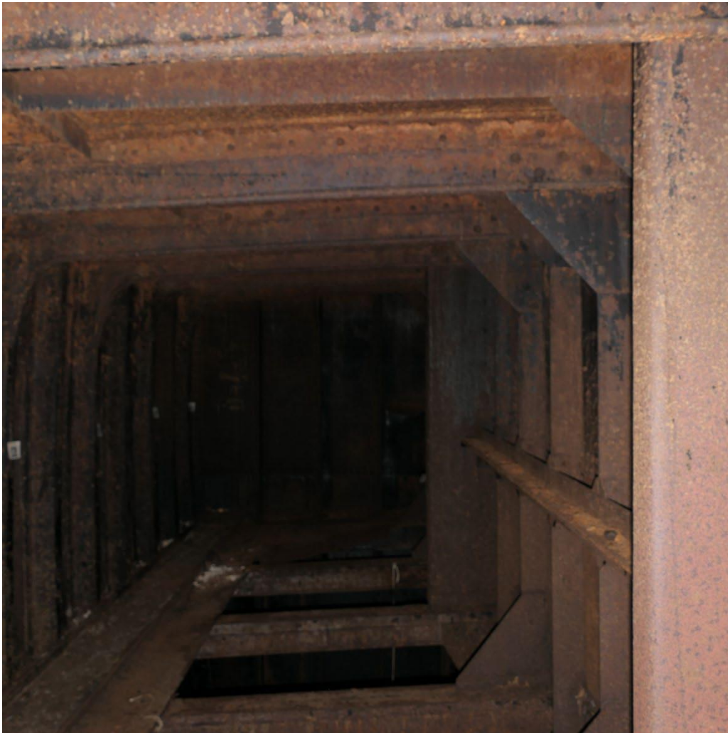
Tank #1, upper flat, looking forward.
