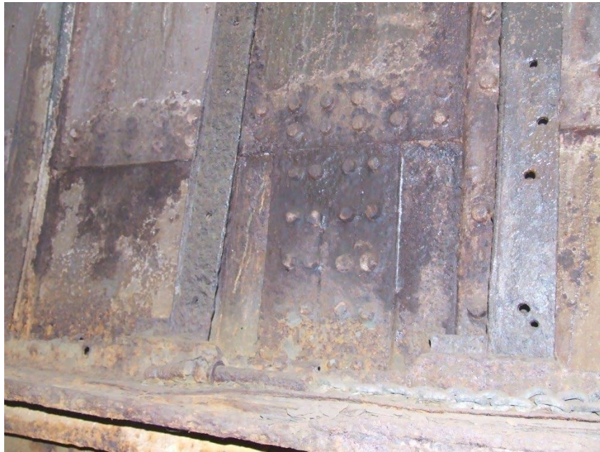
Wasted or non-existent rivets on transverse framing in Pump Room, port side looking aft.
