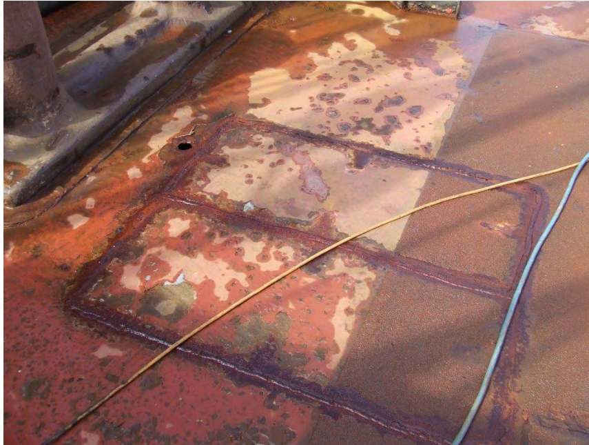
Welded access hatches with failed weldments on main deck.
