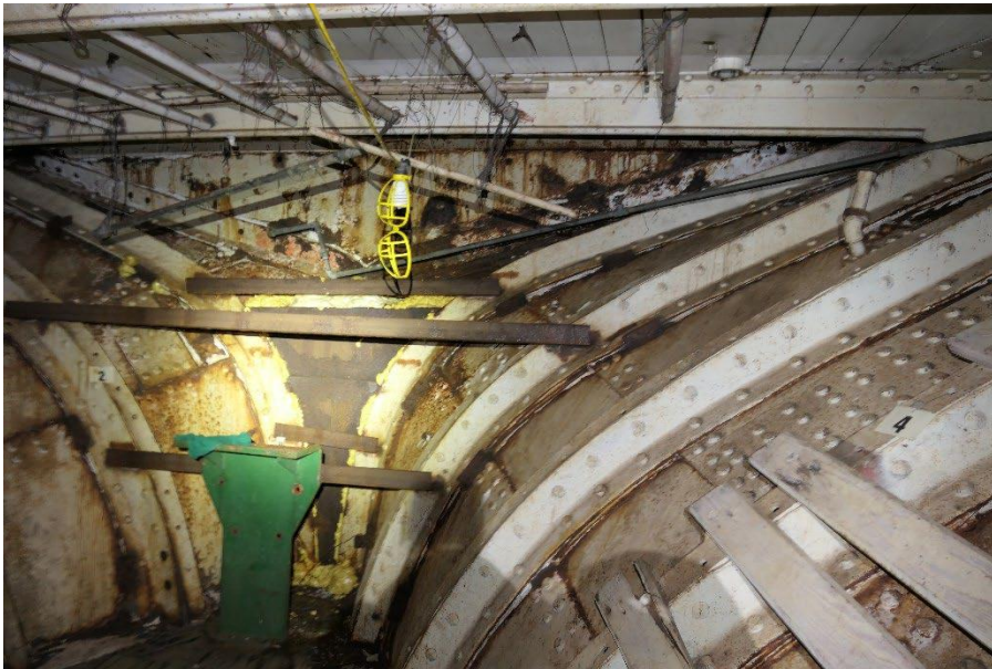
Storeroom at stern, looking aft.. Shell plating separated from frames on both sides leading forward.
