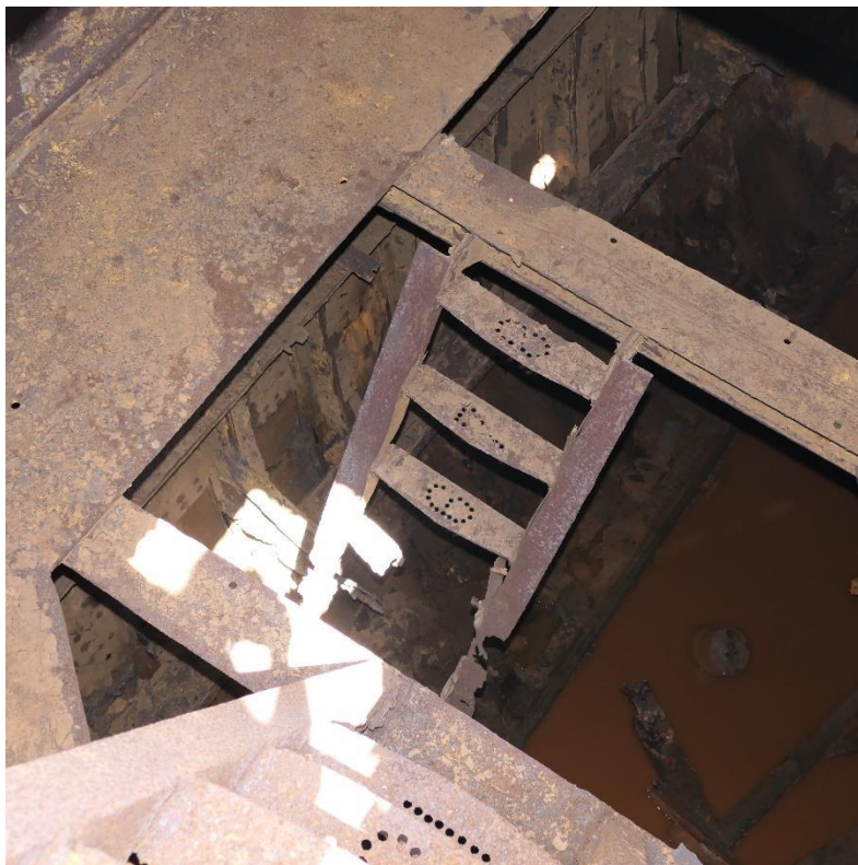
Figure 15: Corroded and partially flooded tank (Joseph Lombardi).
