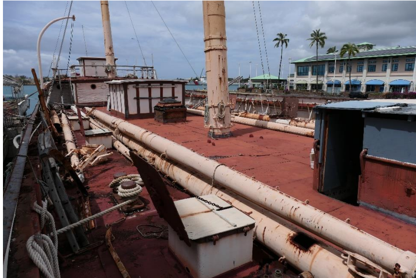
Figure 16: Main deck and aft deckhouses, spars stowed on deck in March 2023 (Joseph Lombardi).
