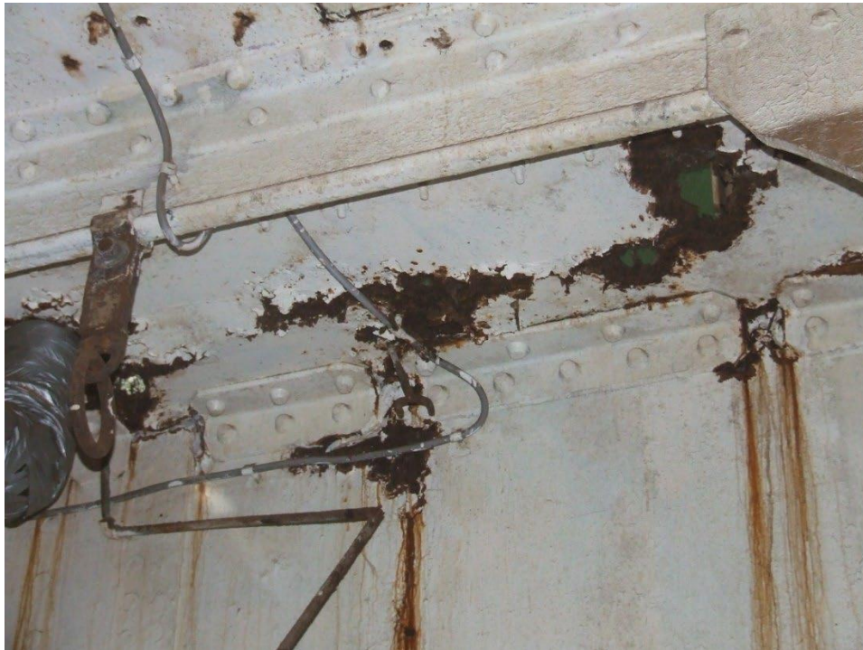
Wasted deck flange on aft bulkhead.
