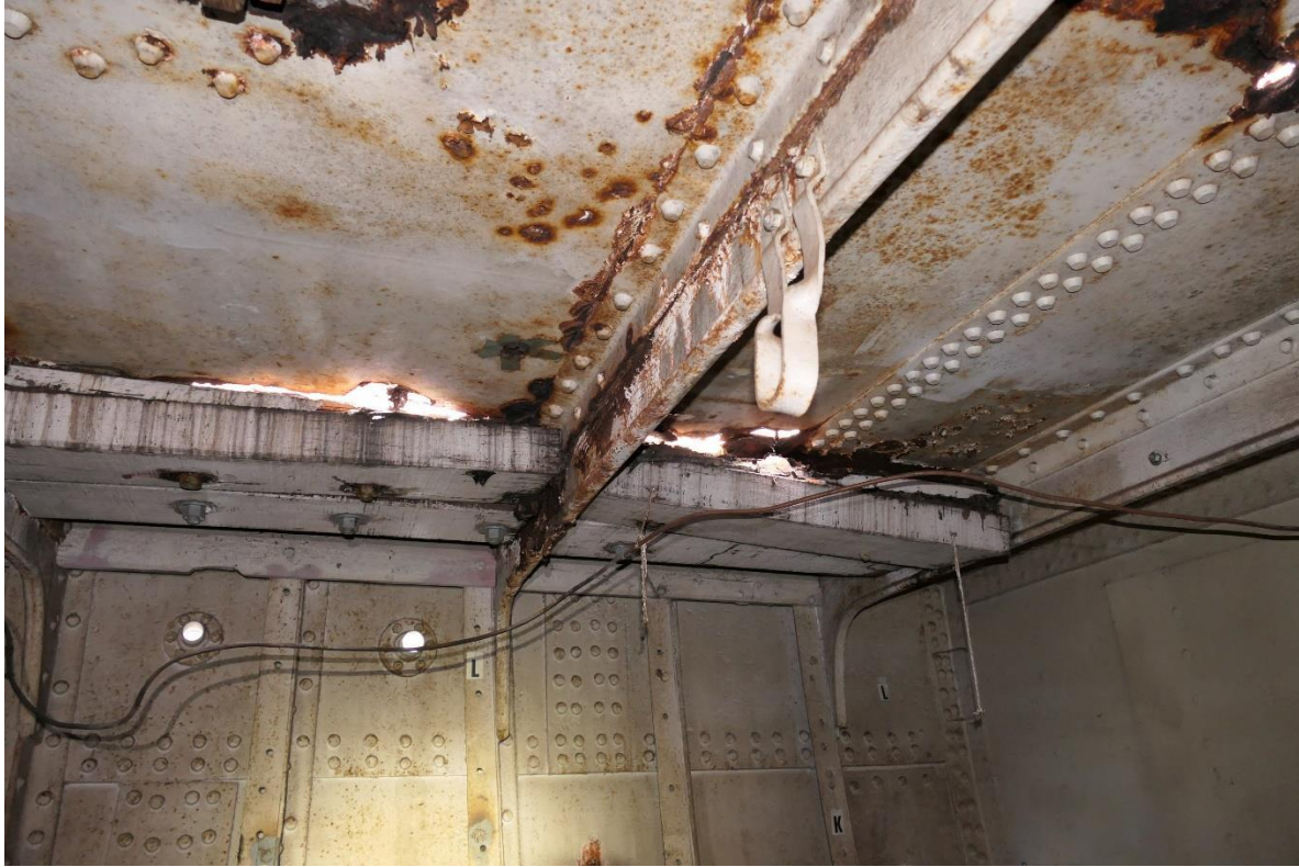
Figure 12: Corrosion has opened holes that have accelerated corrosion inside the ship as well as outside of the vessel (Joseph Lombardi).
