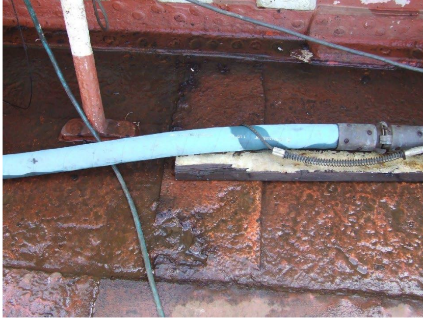
Wasted riveted butt straps connecting deck plating in waterways to port.
