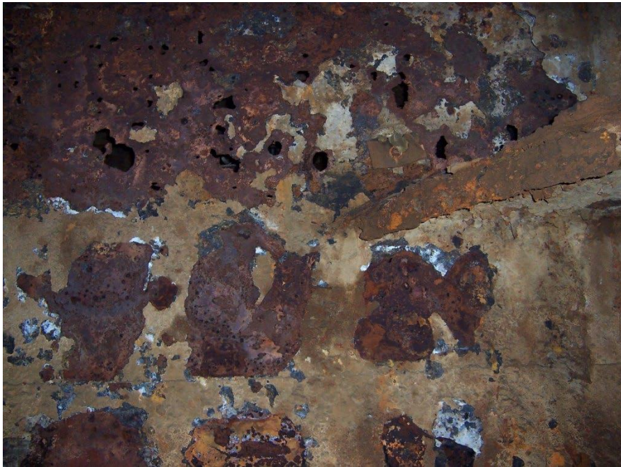
Wasted bulkhead in Tank #1.
