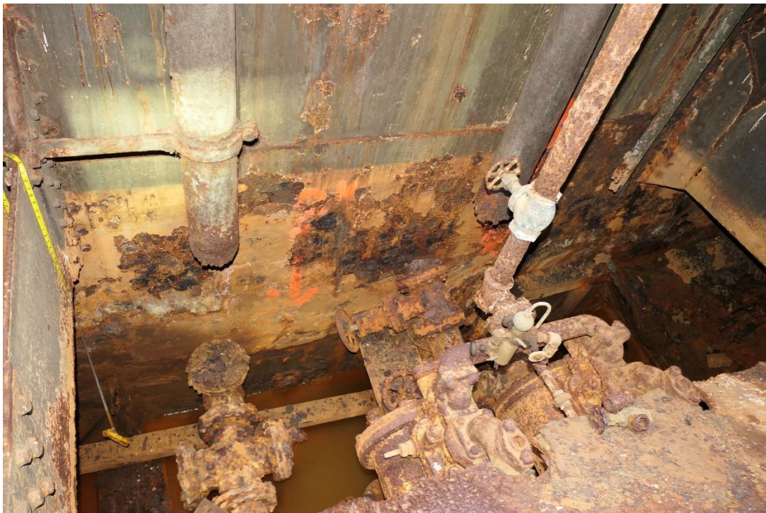
Figure 14: Corroded machinery and piping in 2023 (Joseph Lombardi).
