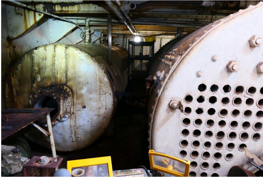
Boiler-room, looking aft to port.
