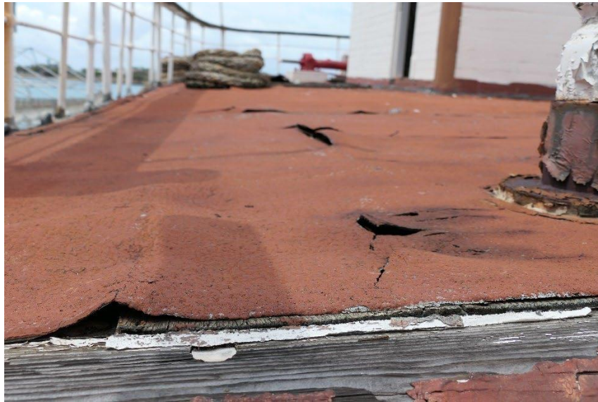
De-laminated sheathing on poop deck.
