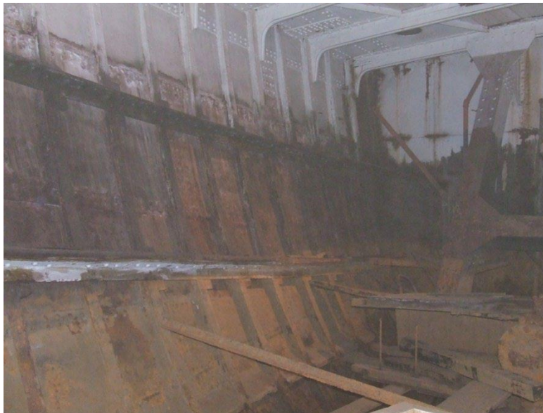
Pump room, looking aft to starboard.
