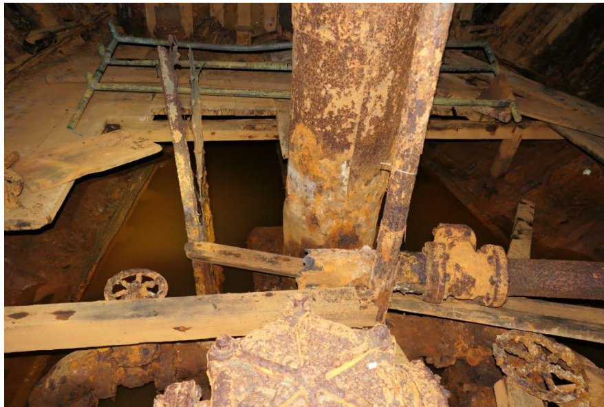
Base of foremast in Pump Room, Heavily scaled.
