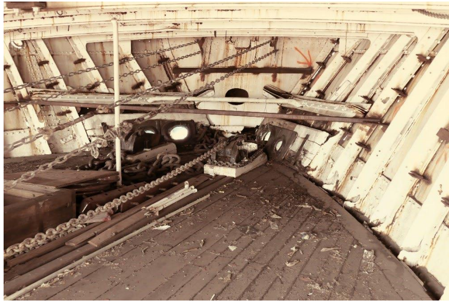
Forecastle showing chains and transverse steel bars supporting collision bulkhead and shell plating to transverse frames.
