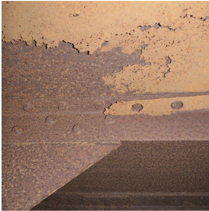
Overhead plate scaling in Tank #3 starboard..
