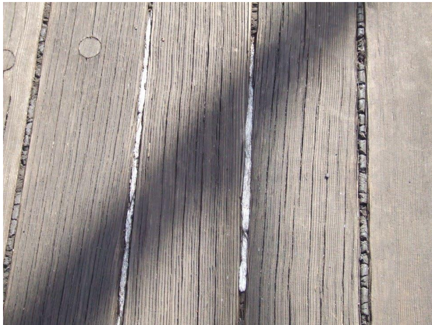
Wasted caulking on wooden decking, notice exposed cotton.
