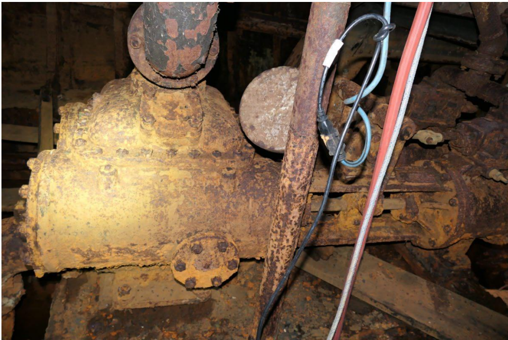
Main steam pump, totally wasted with rust/scale.
