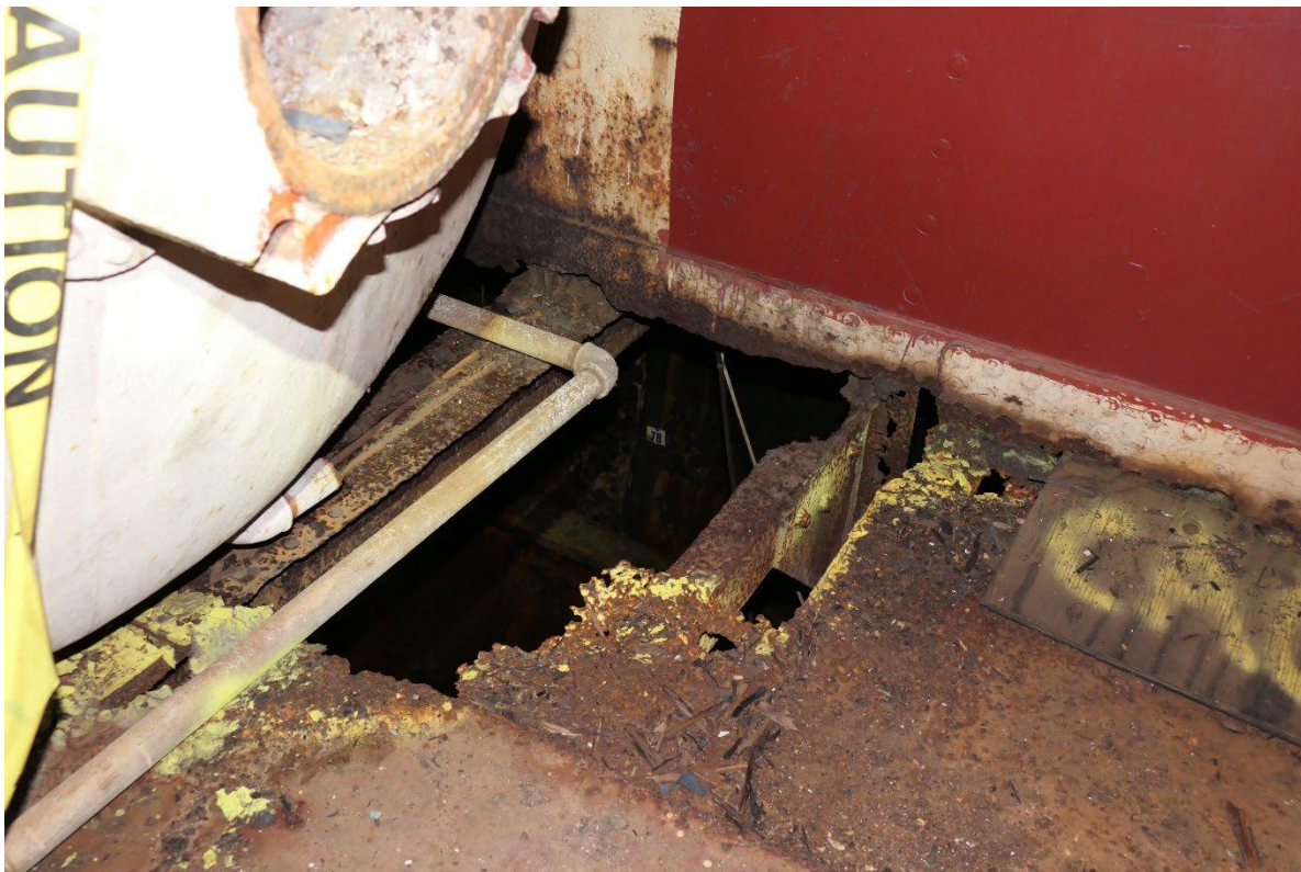
Boiler-room, holed plating to port under boiler.
