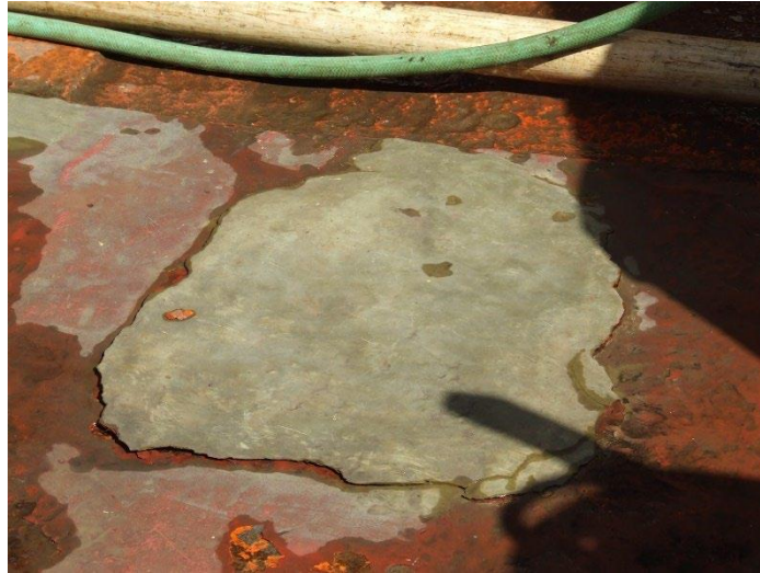
RED HAND epoxy patches that have failed on maindeck.
