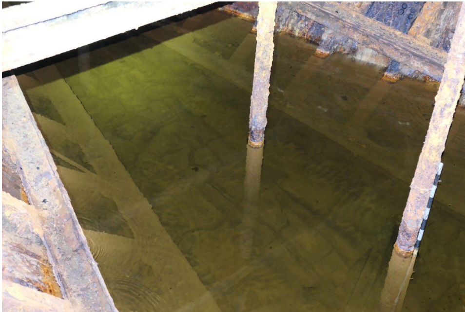
Flooded lower flat of Aft Peak Tank.
