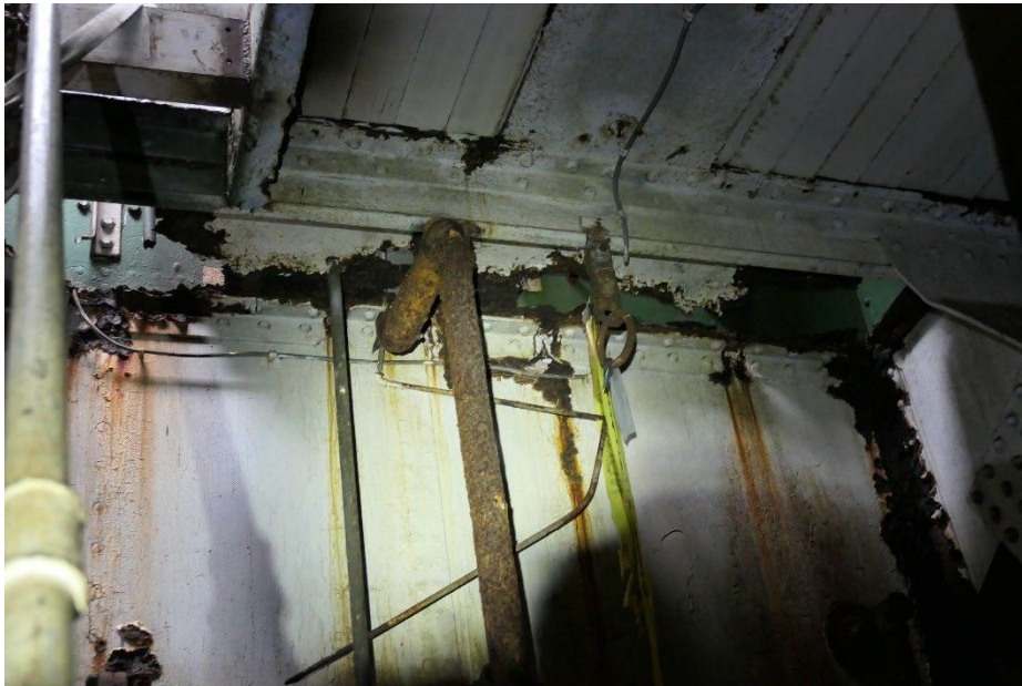
Rotted deck and scantlings at aft end of upper pump room to starboard.
