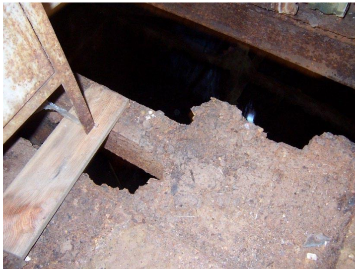
Wasted intermediate platform in Tank #2 port.
