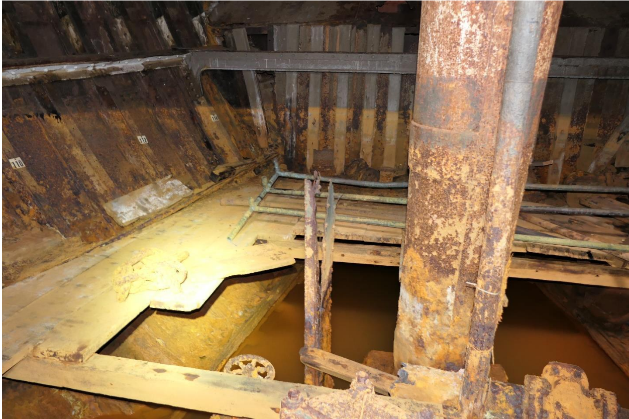
Figure 6: Corroded base of the foremast in the bilge, March 2023 (Joseph Lombardi).
