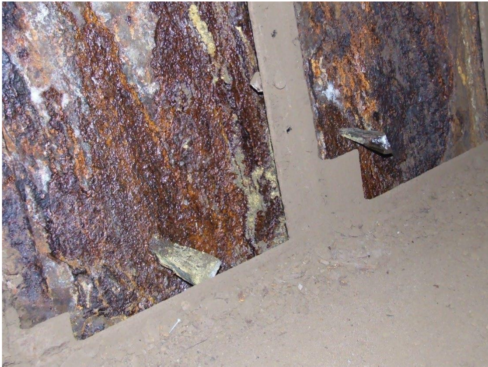
More wasted plating with wooden plugs. Notice separation of shell plating from frames.
