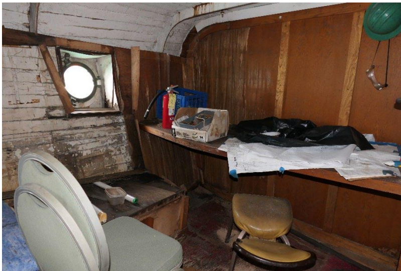
Heavily mildewed hull sheathing with rainwater coming through deck.
