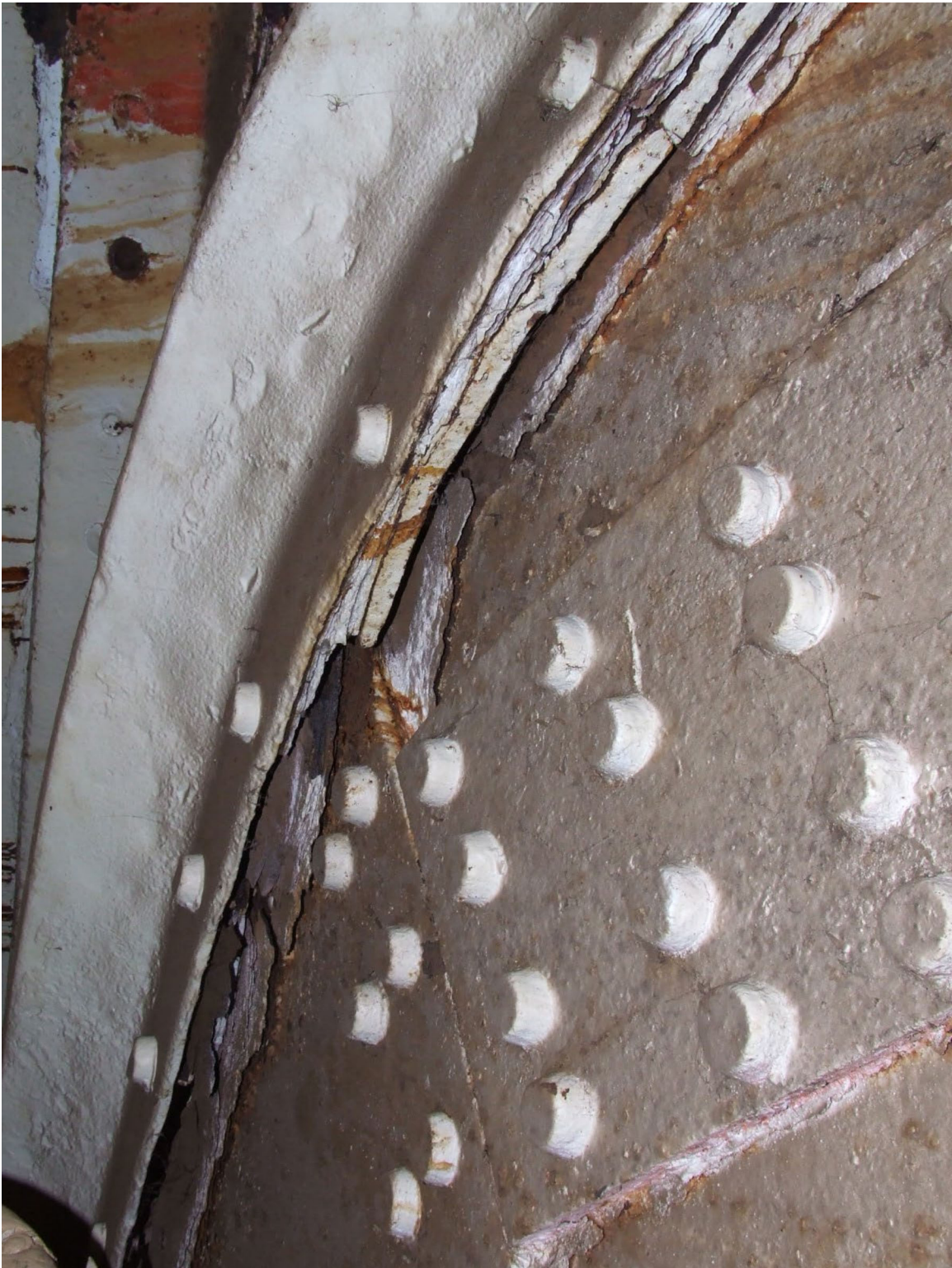
Shell plating detached from transverse frame in Aft Storeroom.
