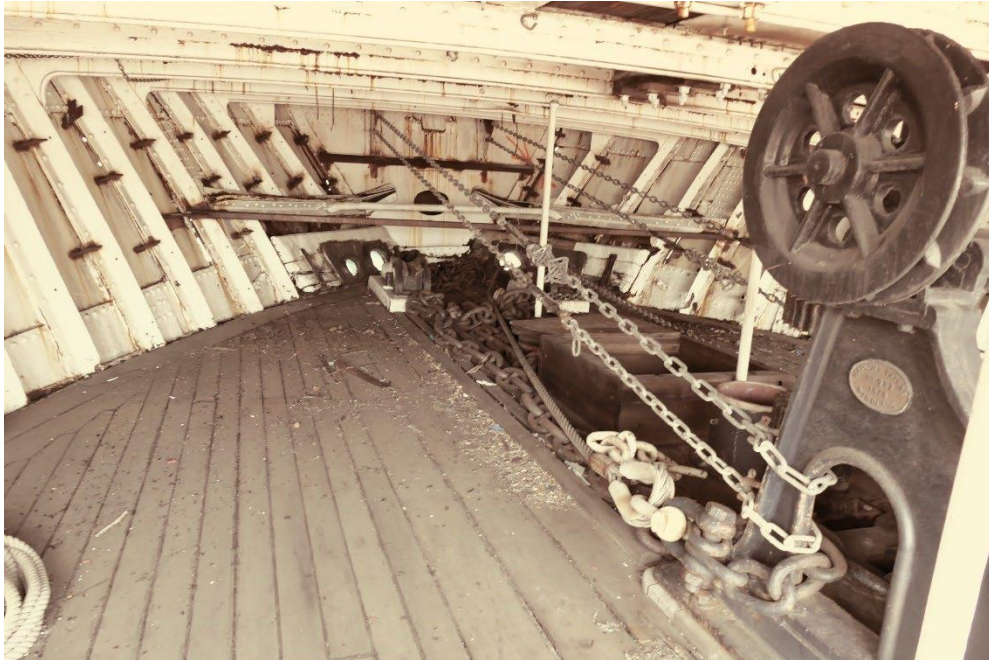
Chains installed in 2008 to support forward collision bulkhead. Transverse steel beams welded across space to pull side shell plating in.
