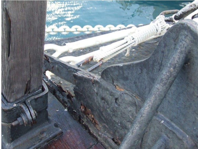
Corrosion of the deck and margin plates is evident in this picture. Notice eyebolt supporting bowsprit guywire lacings.
