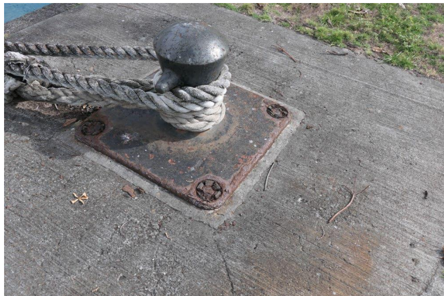
Typical mooring bitt on quay wall with severely deteriorated pins.
