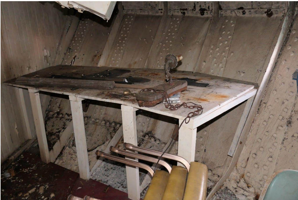
Small cabin to port at the counter showing overhead sagging down at top of photo and poorly maintained inner hull facing.
