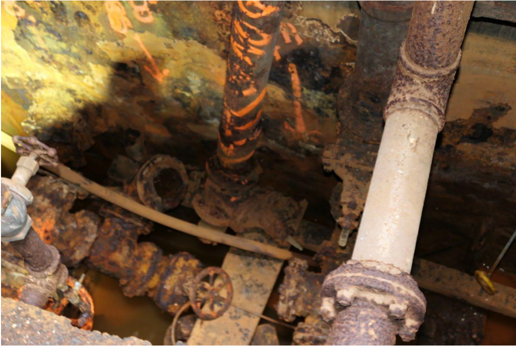
Piping manifold aft of dual steam pumps, showing broken sections in bilges,
