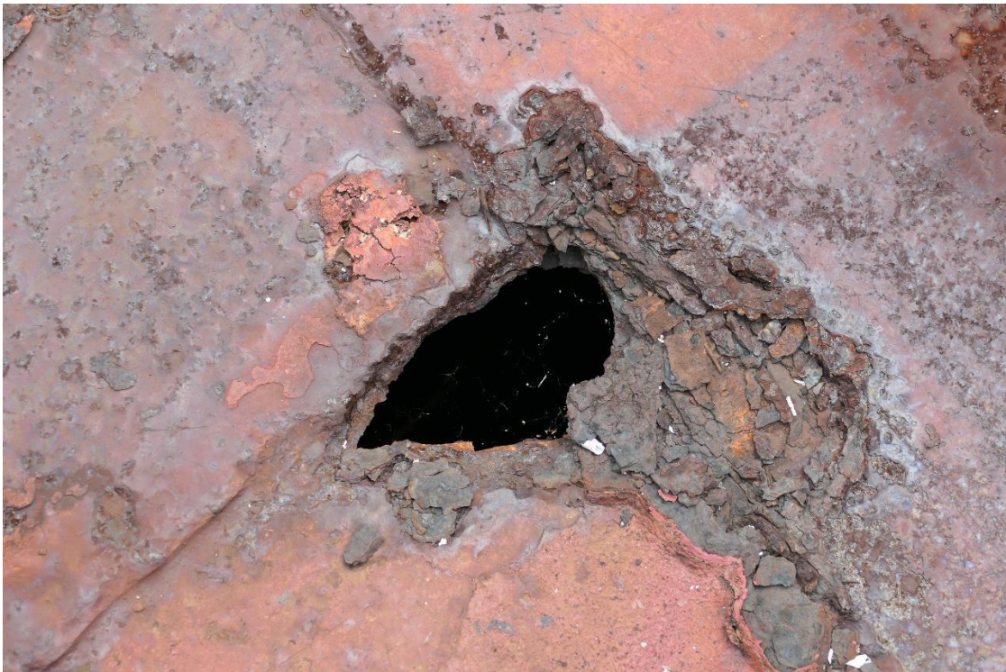
Figure 10: Corrosion has reached the level of complete loss of structural integrity in a number of areas in the hull and decks (Joseph Lombardi).
