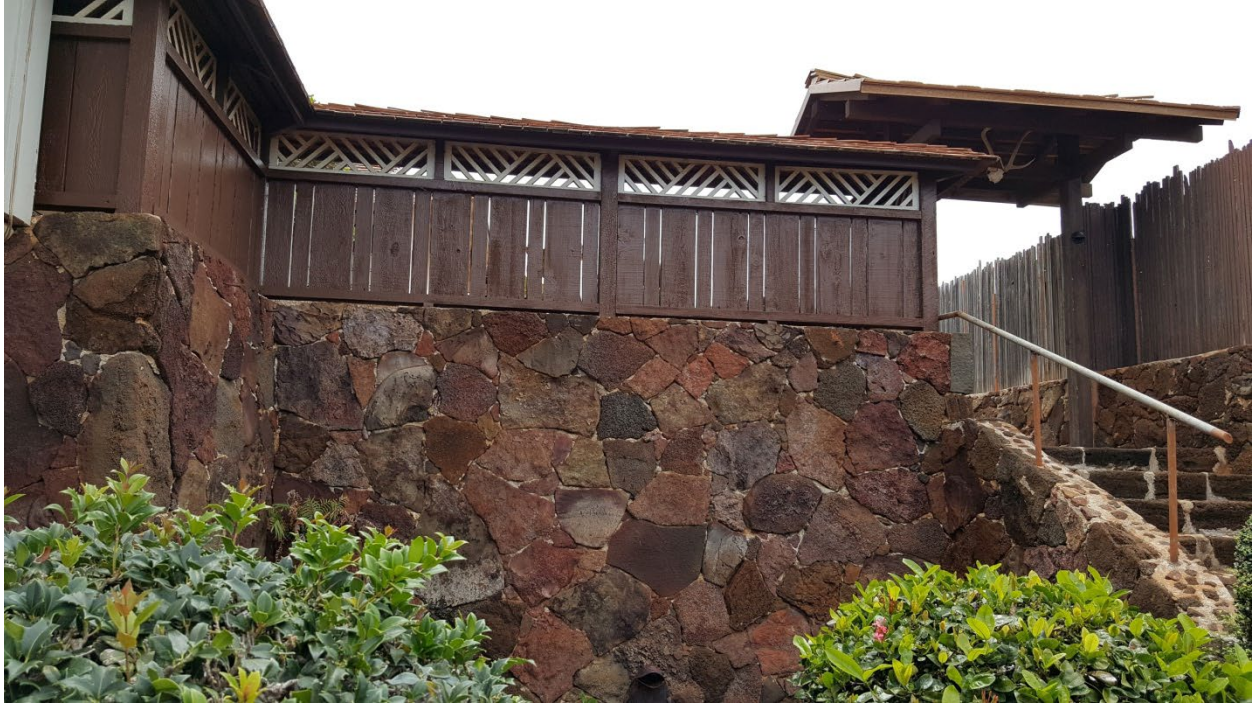
Views of steps and entry gate to third terrace from the east
