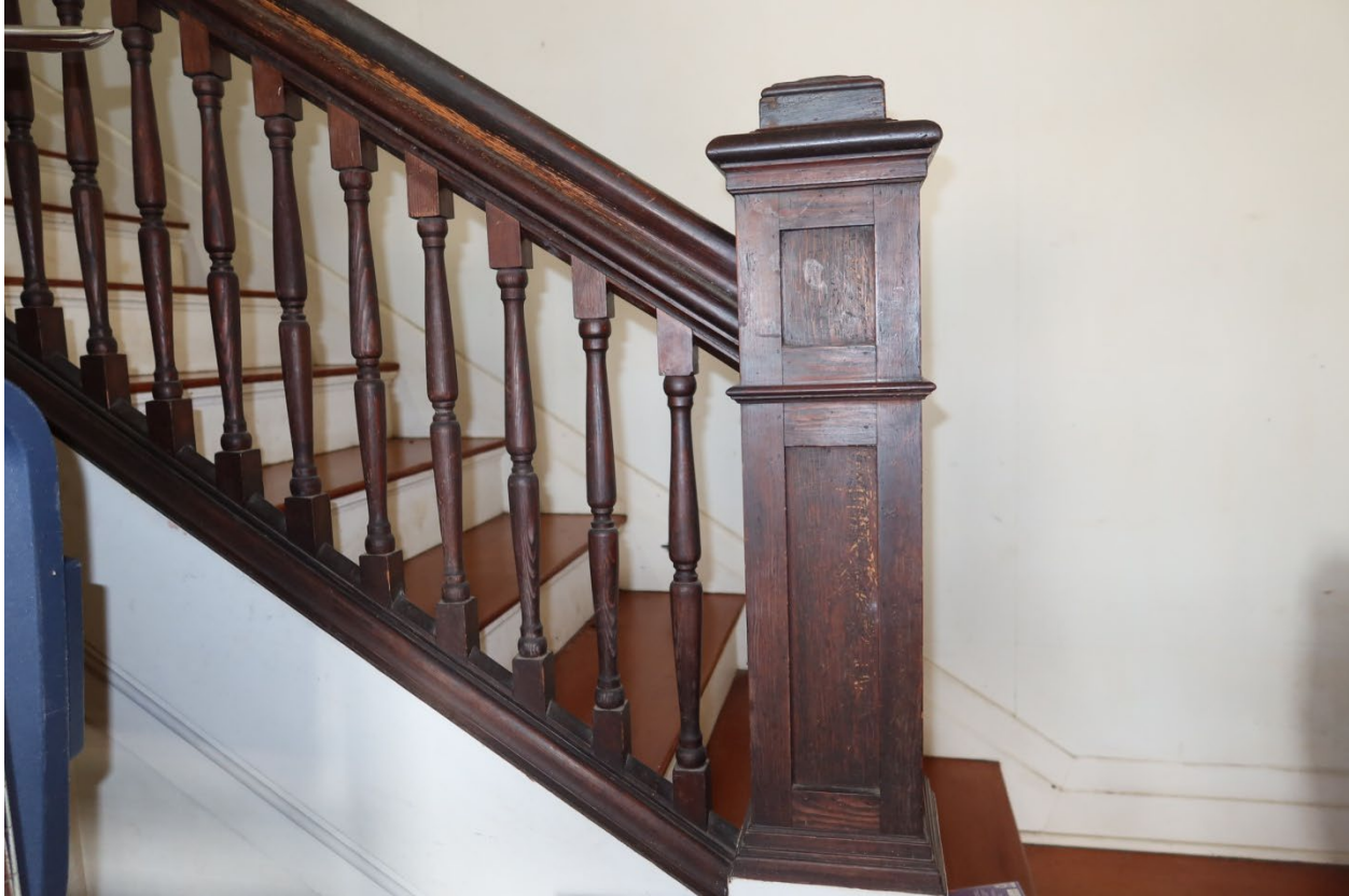
View of the stair's bottom newel post and balustrade from the north
