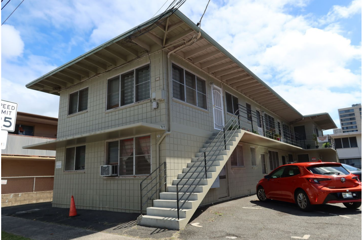
View of the front and side of eight unit, mauka side apartment from the southwest
