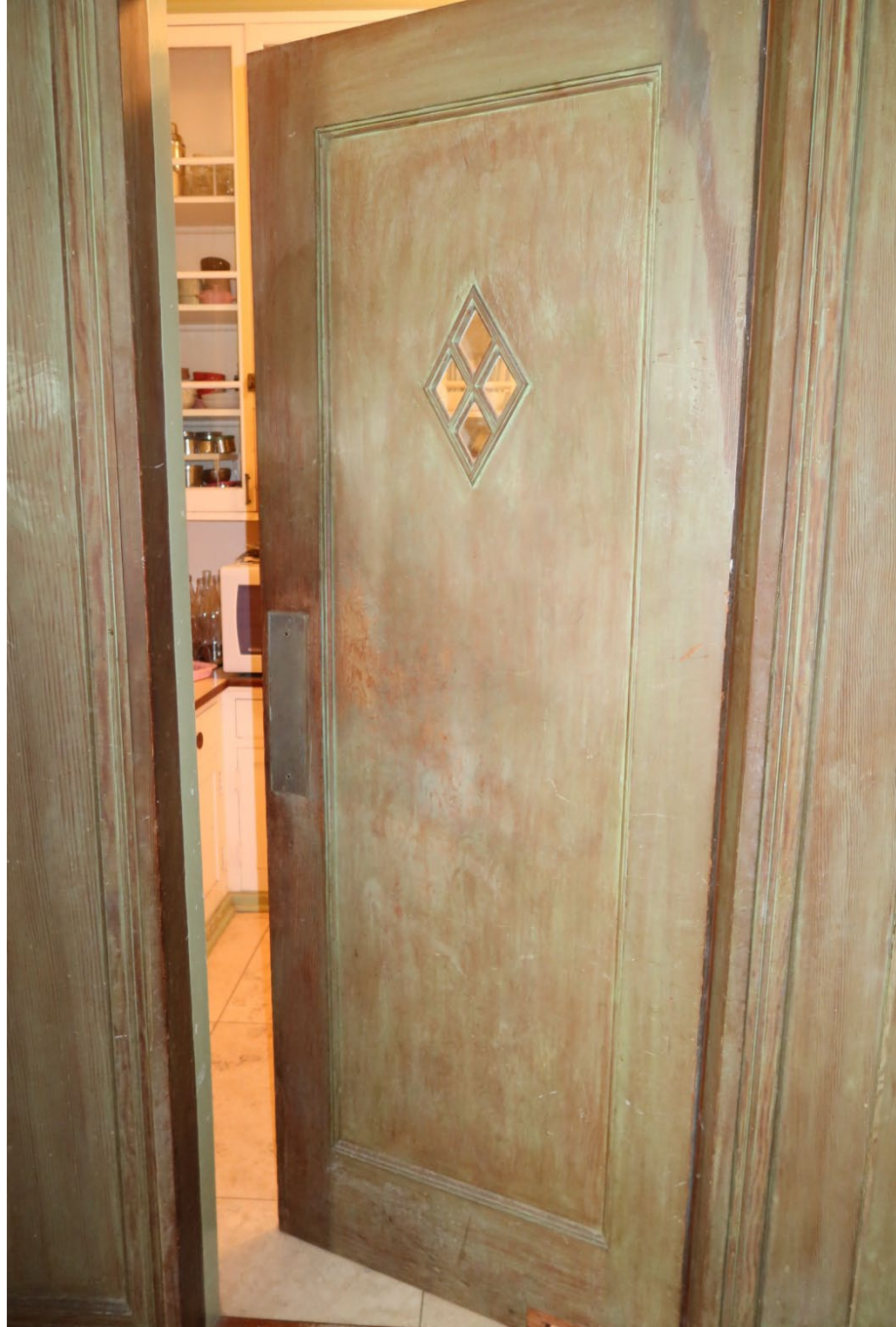
View of door from dining room to butler's pantry from the south
