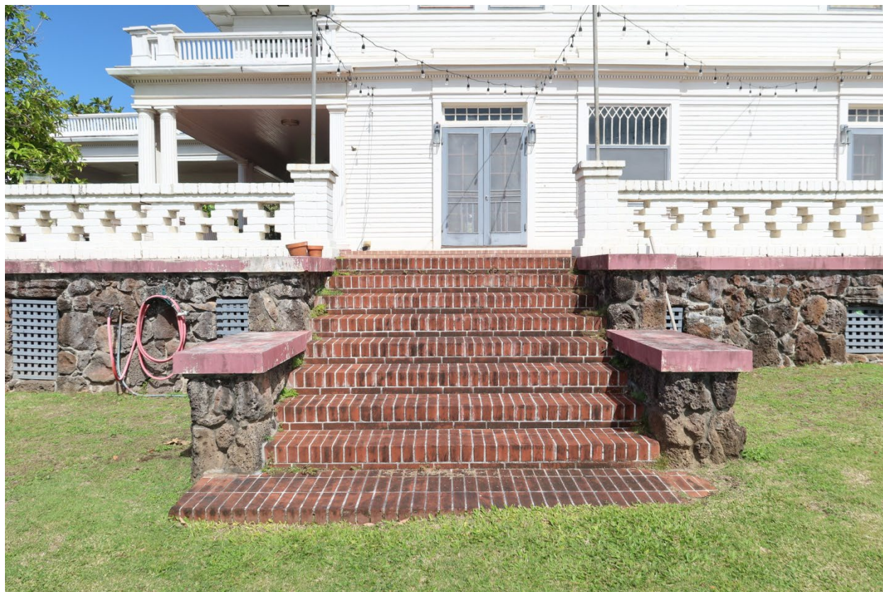
View of steps to patio, patio balustrade and patio entrance to living room from the south
