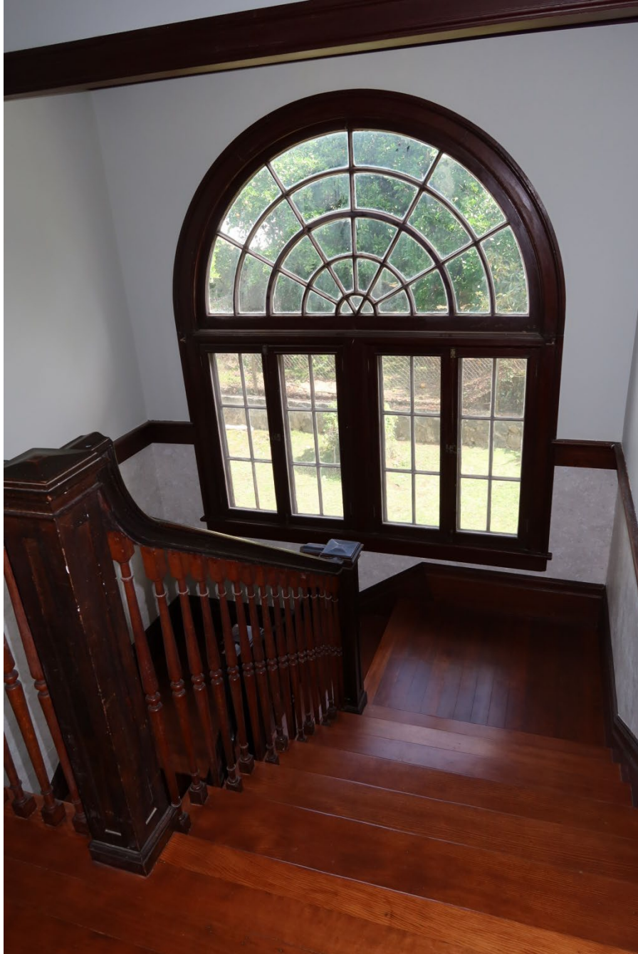
View of casement windows and fanlight at stair landing from the west
