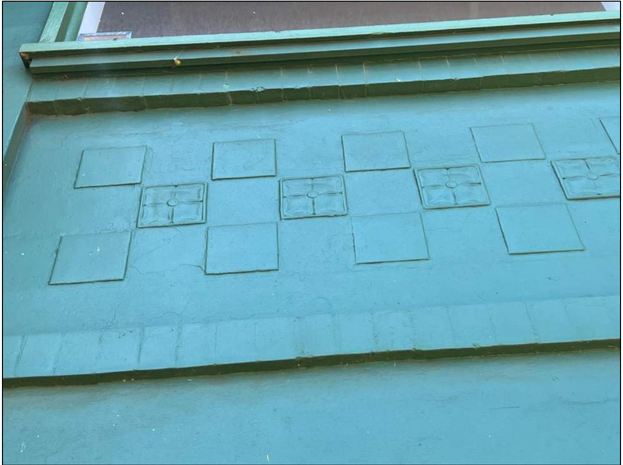
PHOTO 10 Of 18. Old Garage Concrete at House 2 - Tile Detail, North Façade. View to South.
