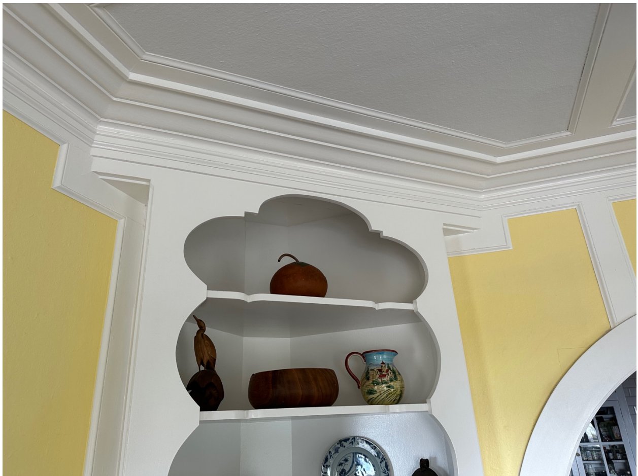
Photo 2 Craftsmanship detail of dining room, showing built in corner cabinet and crown molding.
