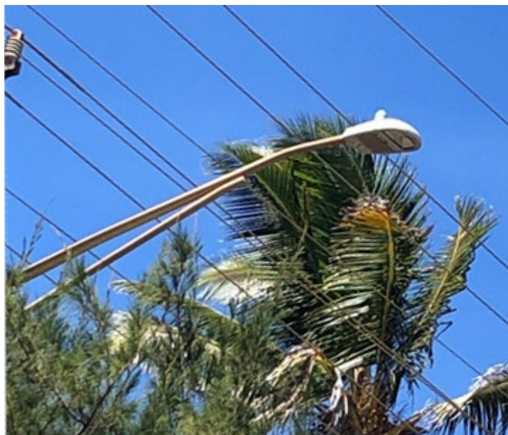
Figure 4-5. Example of Full-Cutoff Shield Installed by KIUC on a Kaua'i Streetlight
