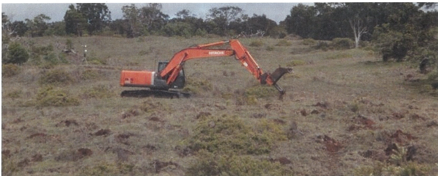
Figure 8. Site preparation methods will include spot cultivation with an excavator in open areas, augmented by manual digging of planting holes in areas with closed canopy forest. Image: K. Derasin 2012.
