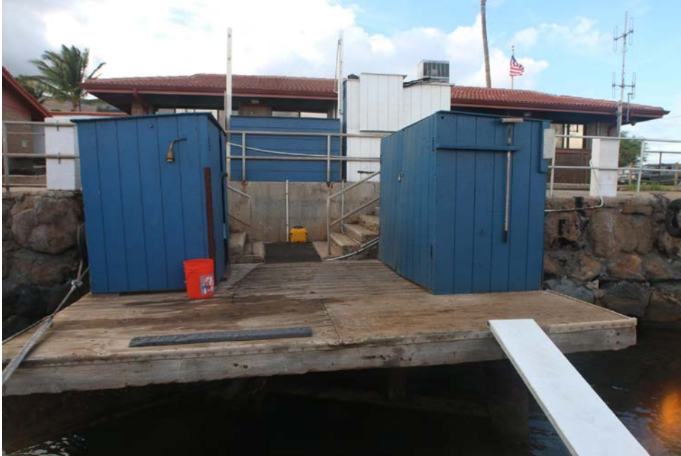
The platform that needs re-decking.
