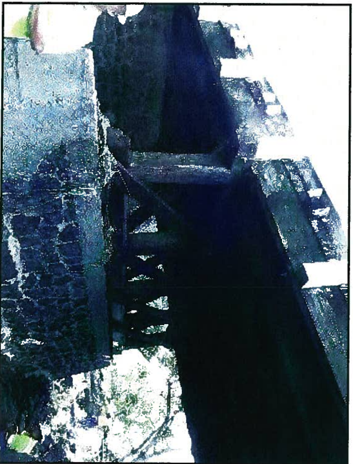
Hilea Bridge timber columns and footings on makai side of bridge, view upstream
