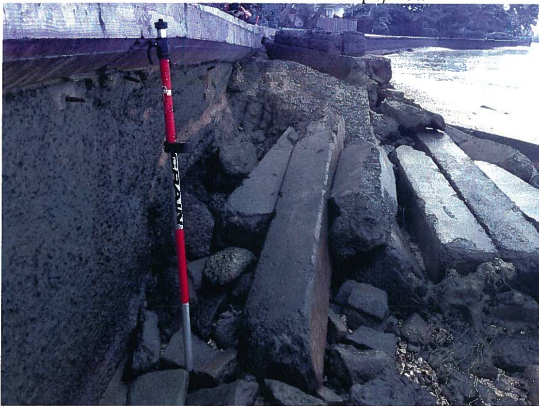
Photo of lip on seawall at project site.
