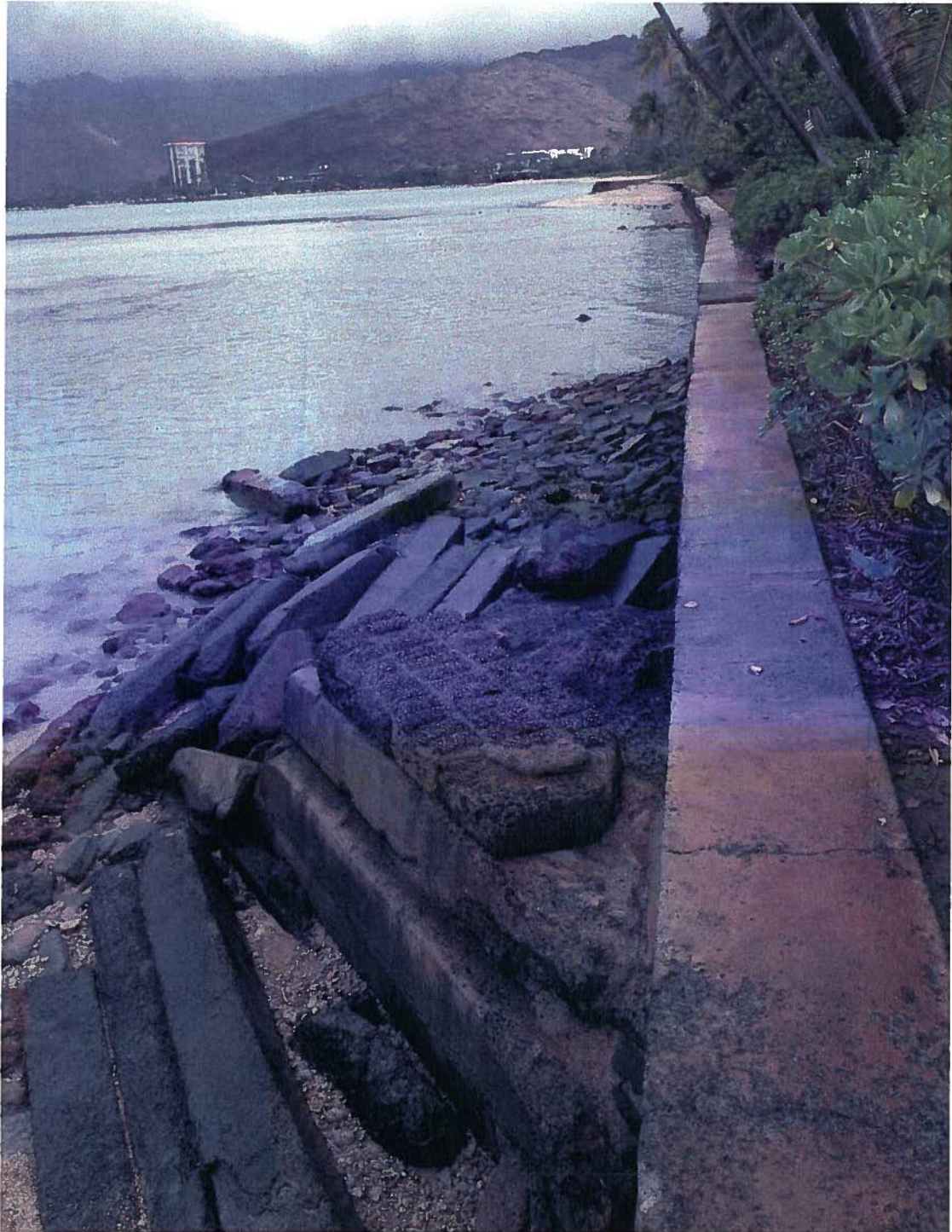
Photo of drainage outlet protection structure with rock debris and piles.
