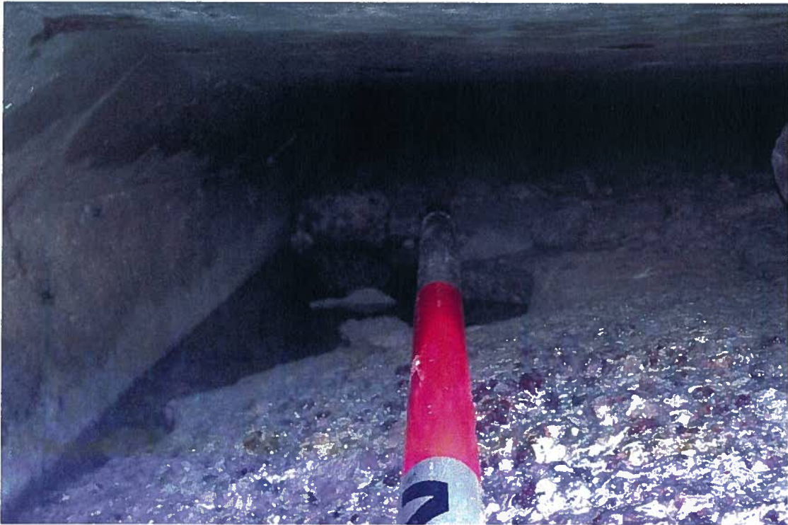
Concrete and debris inside culvert.
