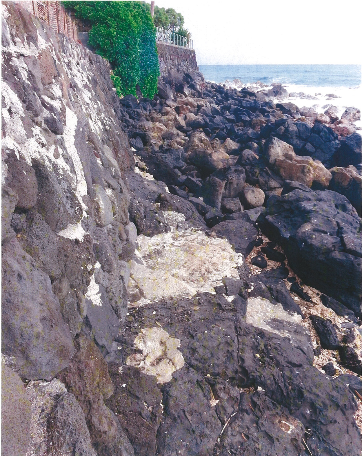
Photo looking east along the face of the seawall. Photo showing concrete fortified rocks in front of the seawall.
