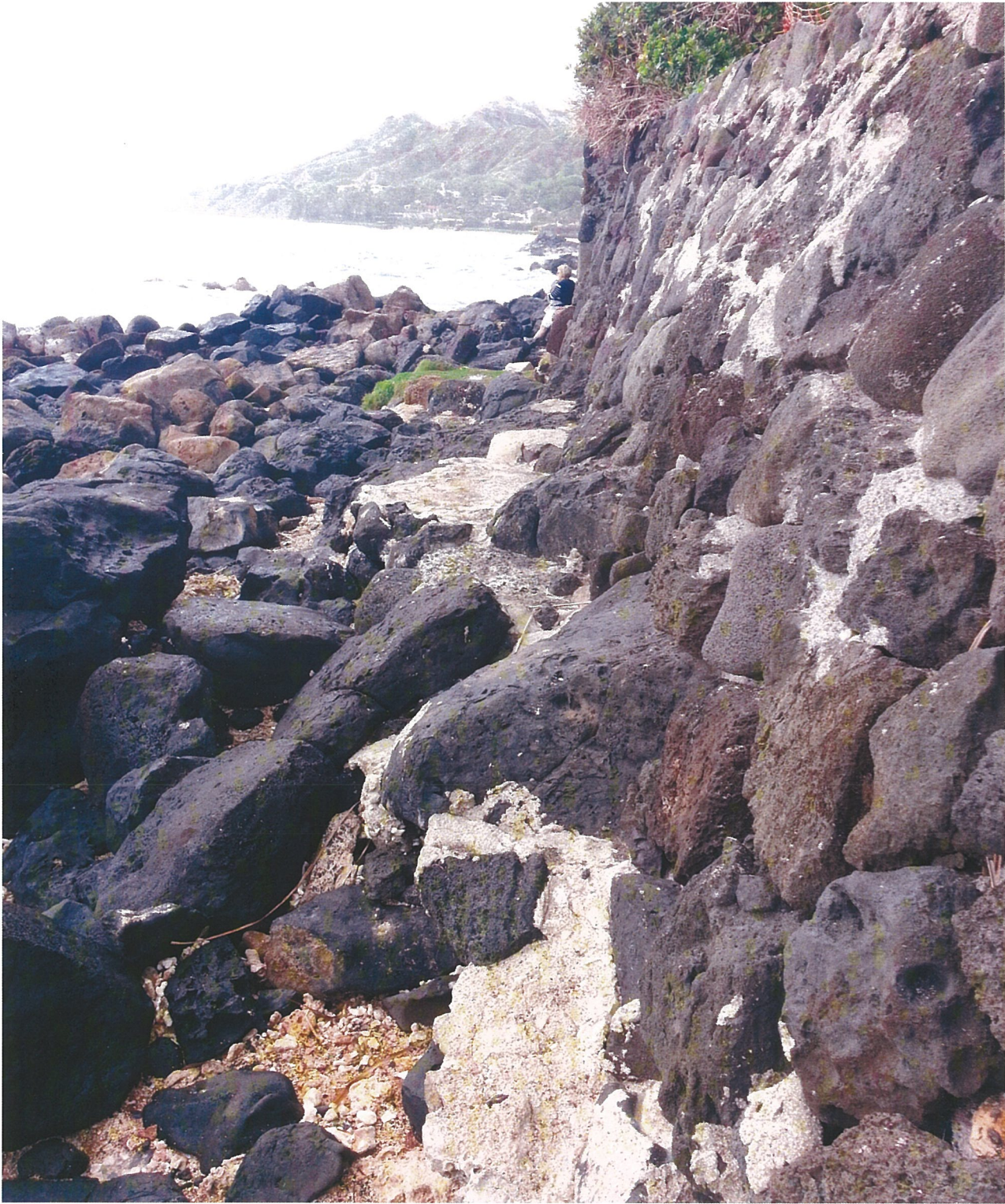
Photo looking west along the face of the seawall. Photo shows encroaching area in front of the seawall with concrete being used to fortify rocks.
