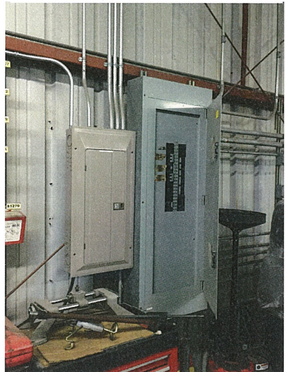
Electrical load center inside smaller bldg
