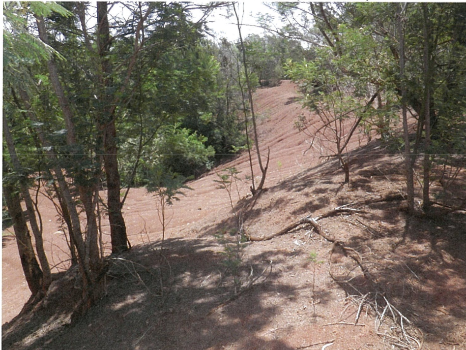
Kitano Reservoir (KA-0004) Trees and Erosion Gullies on the Upstream Slope
