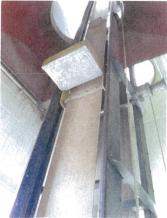
Conveyor belt elevator System from 1 st to 5 th floor
