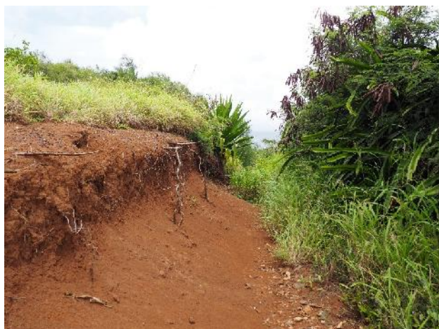
Soils Erosion and Sediment Deposits
