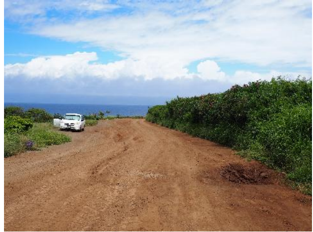
Failed Water Bars
