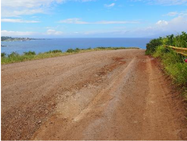
Rills and Channelization
